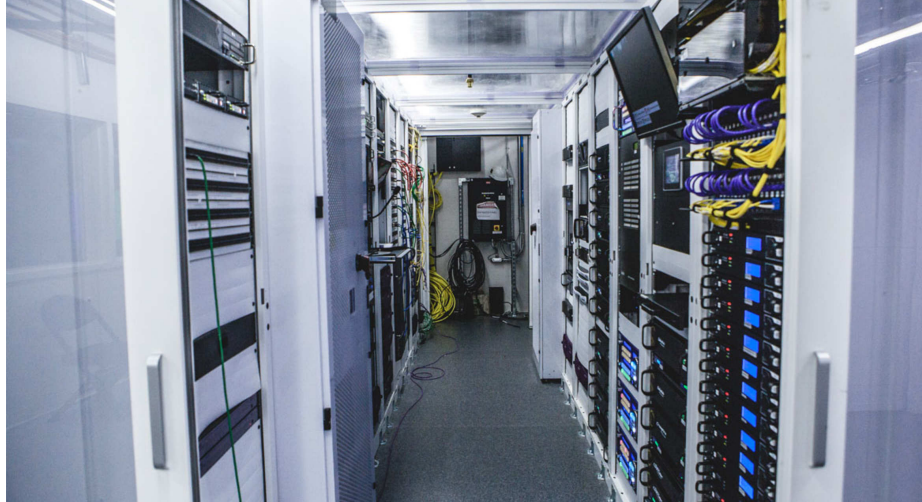
Figure 4.7: The Kings' Golden 1 Center features its own Tier 4 data center, the only one housed inside a professional sports arena (Source: Sacramento Kings).
