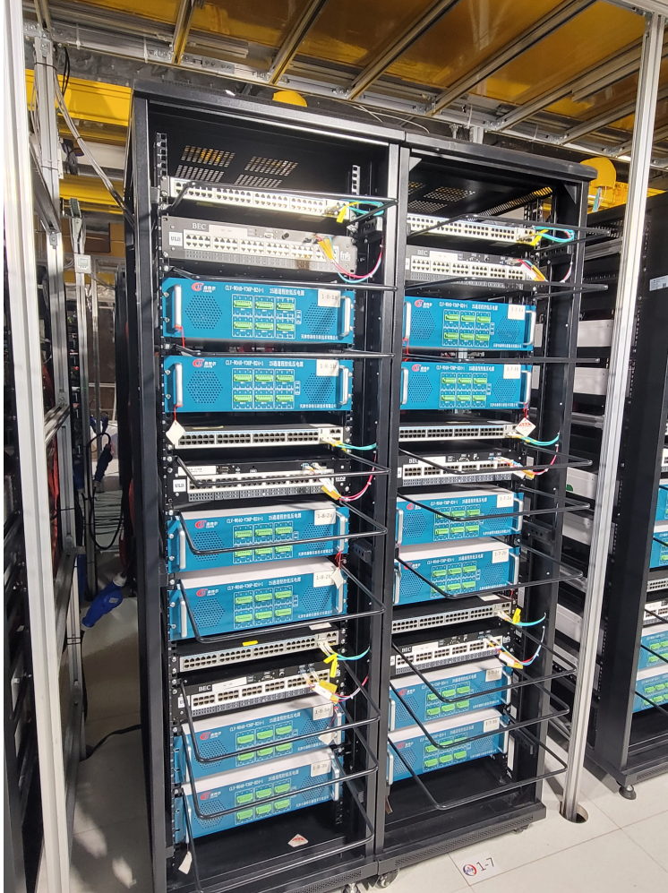
Figure 5.12: JUNO electronics room.
