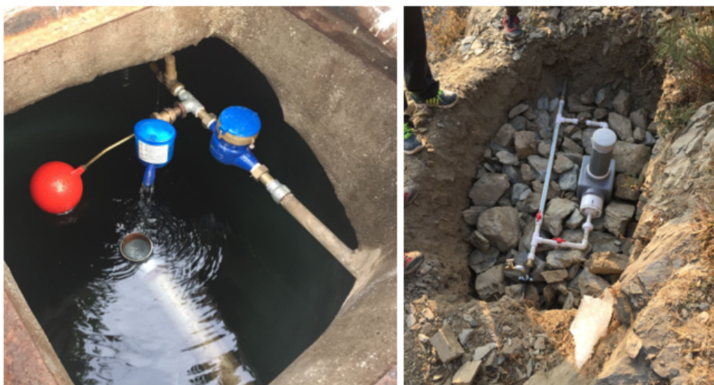
Figure 2.2: Chlorination technologies after installation
