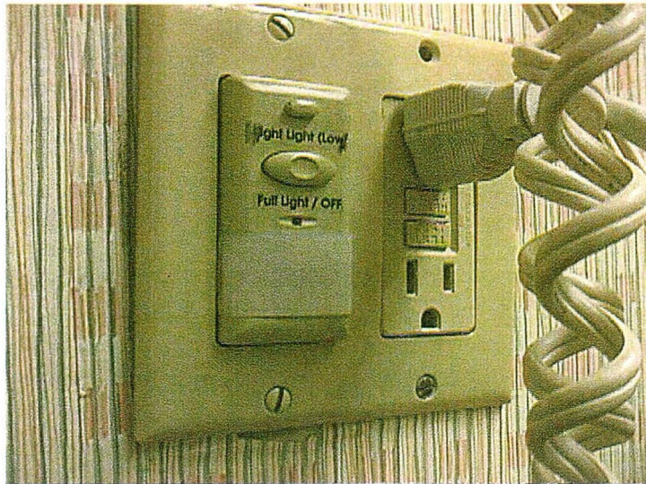
Figure 3: Bathroom controls were co-designed by LBNL and Wattstopper that utilized an occupancy sensor and a low-level “night light” feature.
