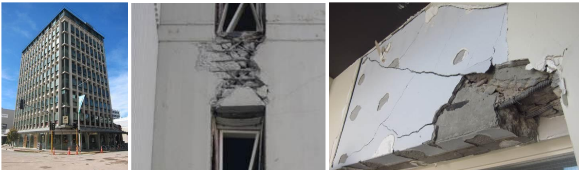
Figure 1-5: Examples of coupling beam damage [11]
