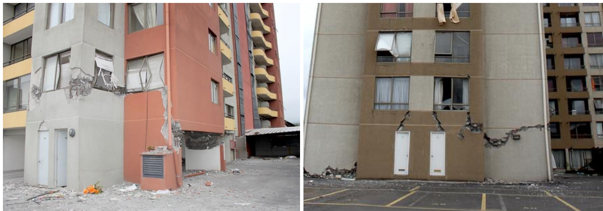
Figure 1-9: Concrete cracking at the base and other stories [37]
