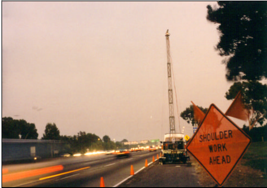
Figure 13.8 Deployment on Road Shoulder, Dusk, US 101, Los Angeles County.
