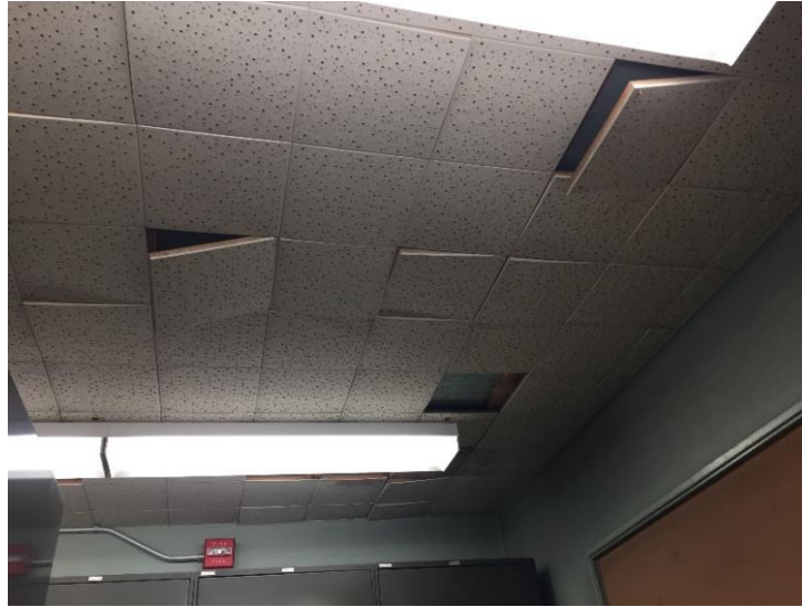
Figure 14. Sagging or missing ceiling tiles on the third floor. This situation is not unique to the herbarium but relatively common throughout the building.
