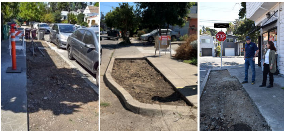
Figure 17: Demolished curbside regions along the block. Credit: Therese Peffer and Haixin Guo
