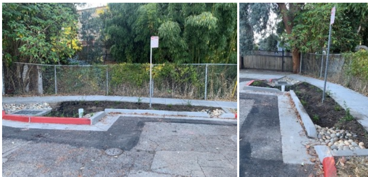
Figure 14: The end-of-block stormwater bioretention facility with local, drought-tolerant plants. Credit: Therese Pepper
