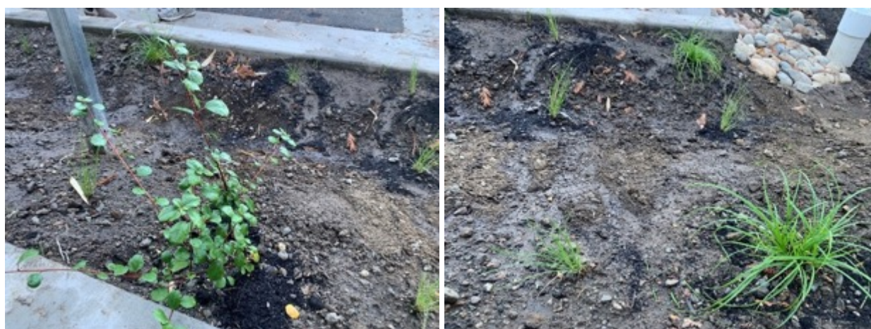
Figure 15: Catalina currant, foothill sedge, and California fescue seedlings were planted in the stormwater bioretention facility. Credit: Therese Pepper
