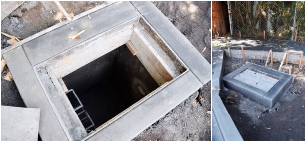
Figure 10: The stormwater drain in the facility. Credit: Haixin Guo
