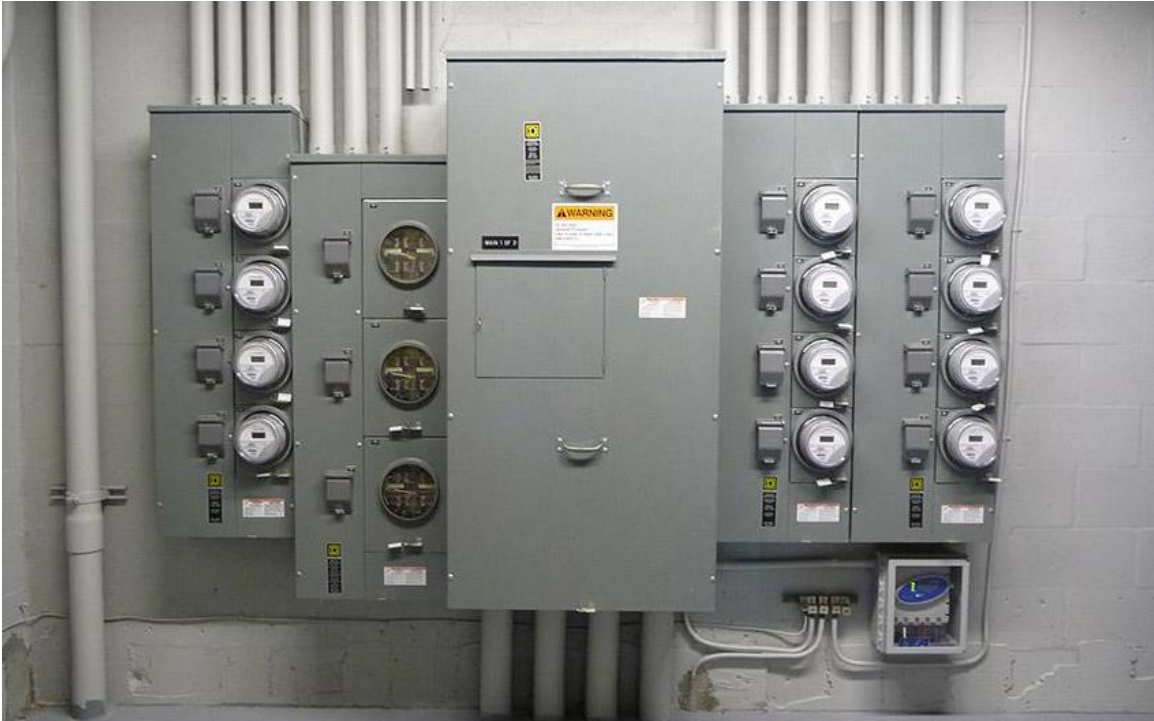
Figure 3: Image of a load center at a typical mid-sized multi-family property with separate sub-panels for each dwelling unit as well as building-wide communally metered loads.
