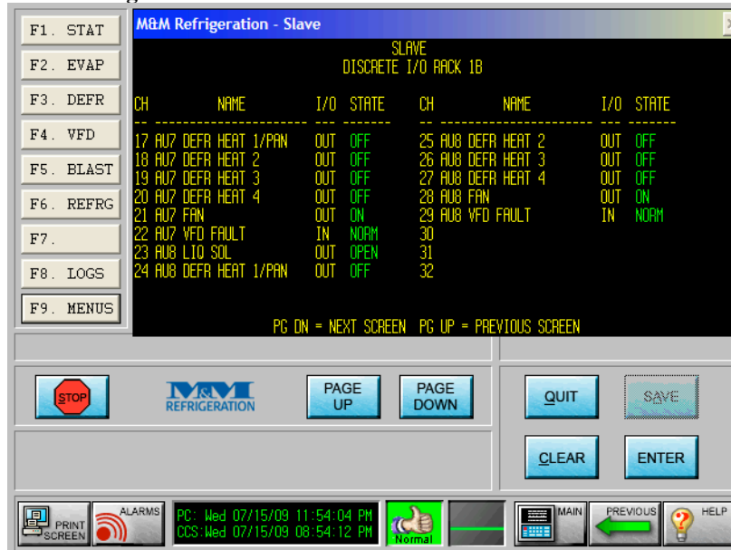
Figure 9: Installed Slave Panel Discrete I/O Rack 1B
