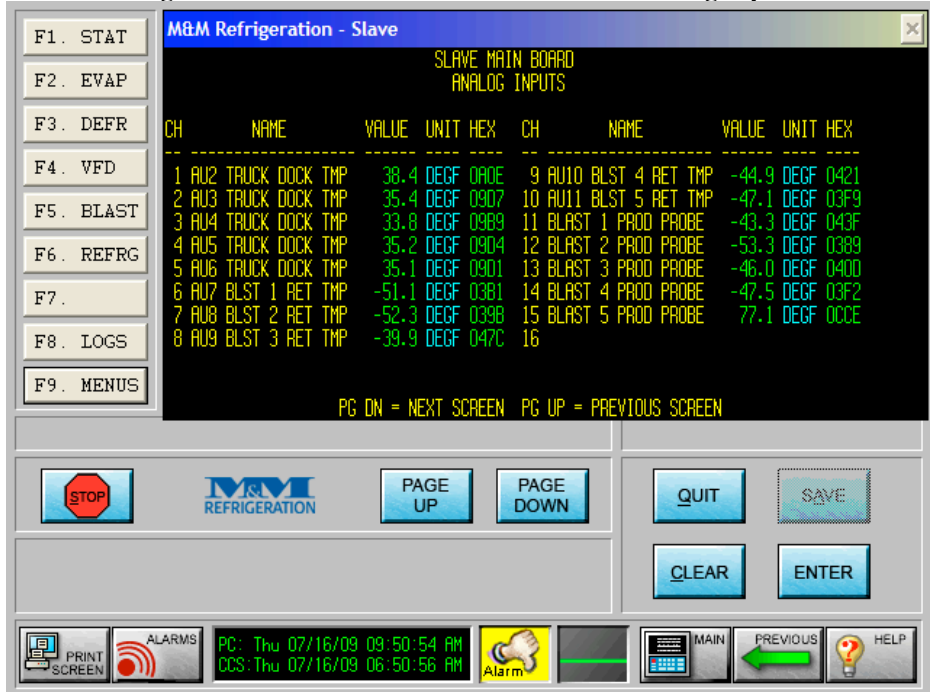
Figure 7: Installed Slave Panel Main Board Analog Inputs
