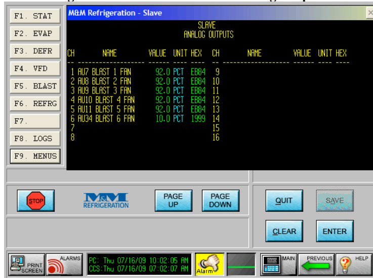
Figure 6: Installed Slave Panel Analog Outputs
