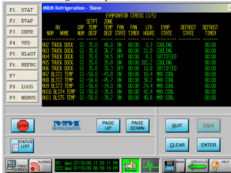
Figure 5: Evaporator Status Screen
