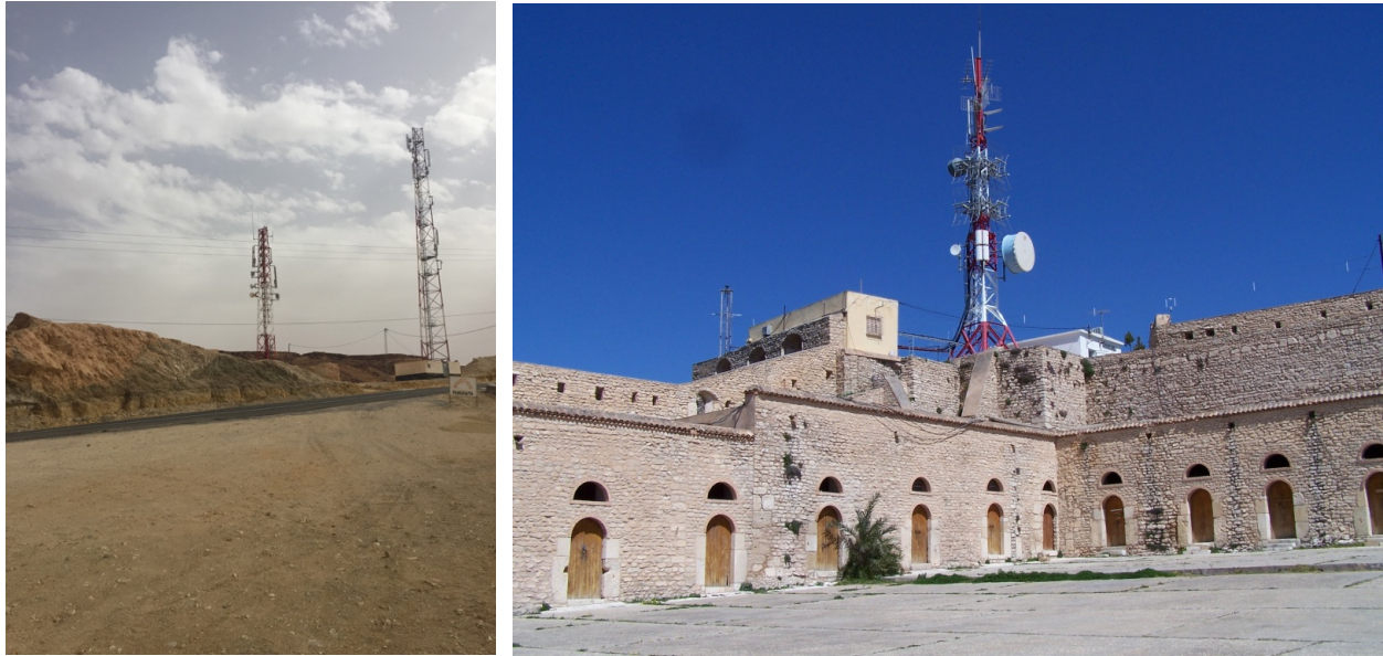
Figure 2 Transmission towers in the rural interior (left) and within the Ottoman fortress in El Kef (right). Photographs by the author.
