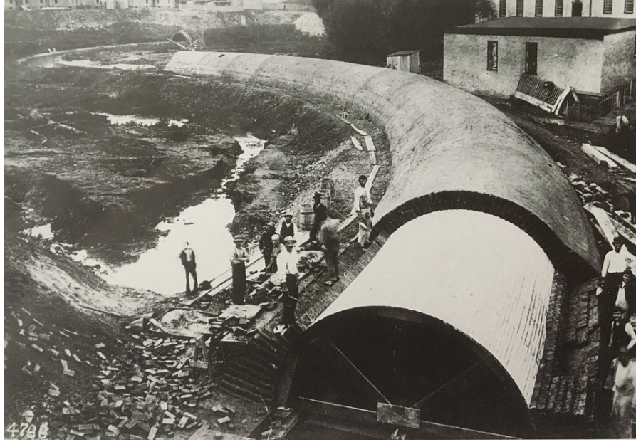
Above: The Undergrounding of Mill Creek in 1880s Western Philadelphia. Shunting stormwater into a massive culvert beneath the town caused extensive, multi-generational problems, and entailed an impressive earthmoving enterprise to accomplish in the first place. Note the sheer displacement of earth by the structure; and the volume required to eventually re-establish grade above it. Philadelphia Water Department
