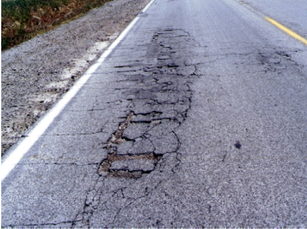
Figure 1. Typical distress visible on State Route 138.
