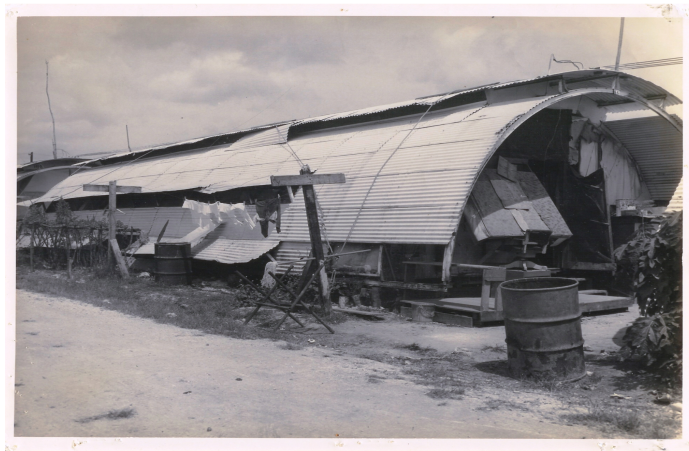
Figure 3.6 Outside Condition of a Damaged Quonset hut at Camp Roxas. Source: Guam Humanities Council
