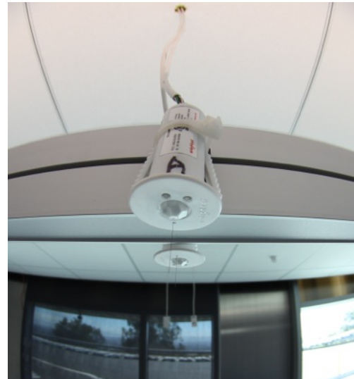
Figure 5.3 - Two Enlighted sensors attached to one Vode light fixture. The sensors were adhered to the side of the fixture because sensor integration hadn’t been coordinated between manufacturers yet.
