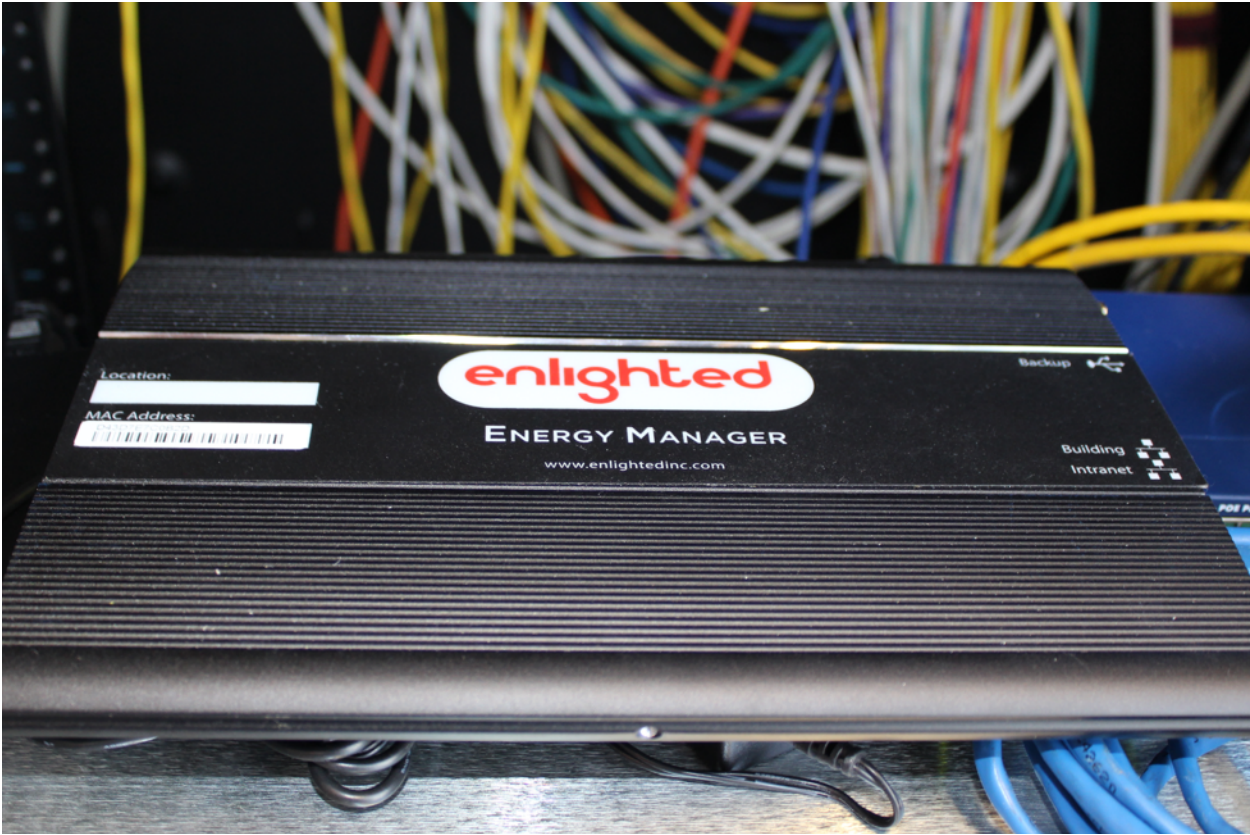
Figure 5.1 - The Enlighted energy manager located in the server closet.
