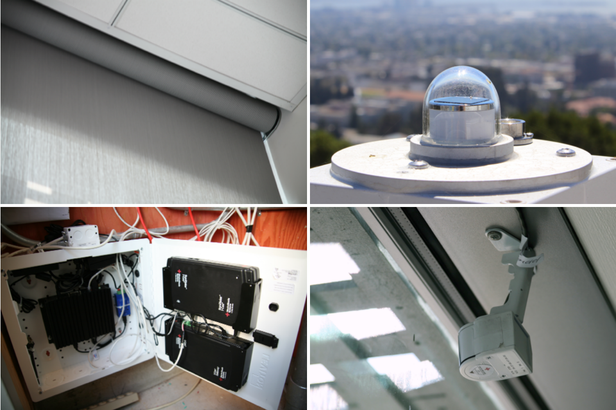
Figure 7.1 - Photographs of MechoSystems components. Clockwise from top left: motorized roller shade (medium grey color), rooftop irradiance sensor, illuminance sensor mounted to the window frame, MechoSystems control cabinet.
