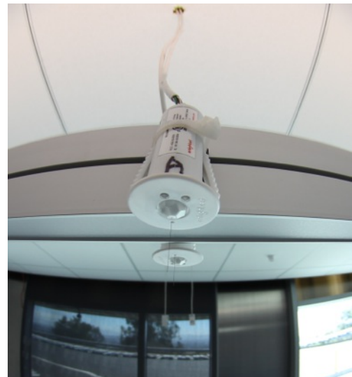
Figure 5.3 - Two Enlighted sensors attached to one Vode light fixture. The sensors were adhered to the side of the fixture because sensor integration hadn’t been coordinated between manufacturers yet.
