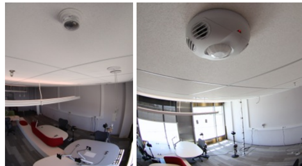
Figure 4.3 - Encelium photo sensor (left) and occupancy sensor (right) installed in FLEXLAB.
