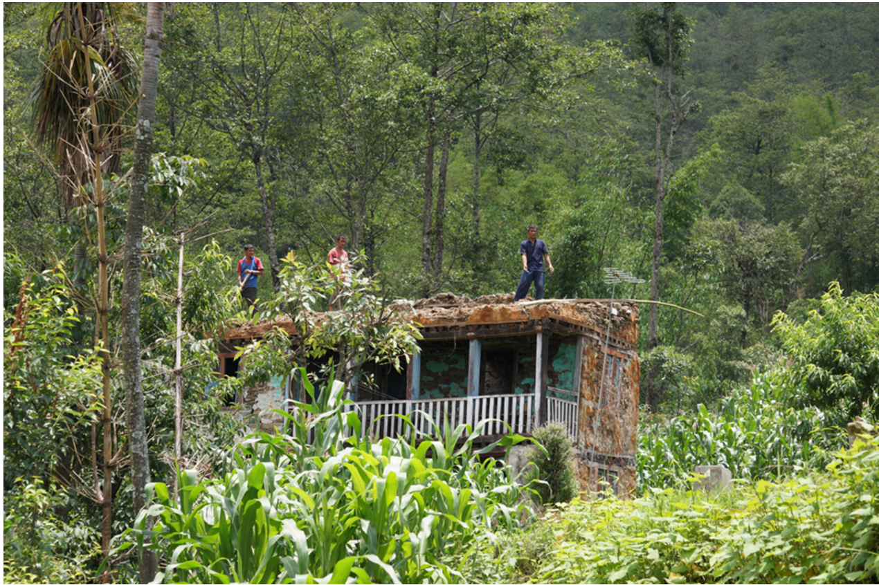
FIGURE 8. Photograph of neighbors assisting with repairing damaged farmhouse. Farmers reported that in the days immediately following the earthquake, friends and neighbors as well as representatives from local institutions like community forestry groups, were among the first to respond. These types of practices build post-disaster resilience.
