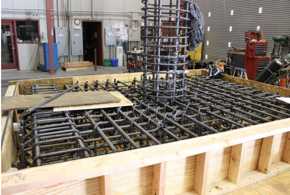
Figure 5.12 – Picture of the slab and column reinforcement of Specimen #1 prior to cast
