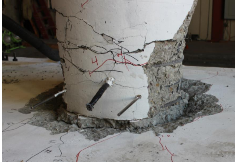
Figure 5.37 – Damage at the slab-column interface after the testing of Specimen #3
