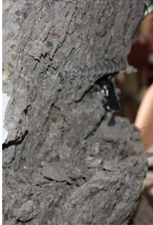
Figure 3.33 – Buckled Bar 1 at south face of Specimen #1 during 2 nd cycle of -8% drift
