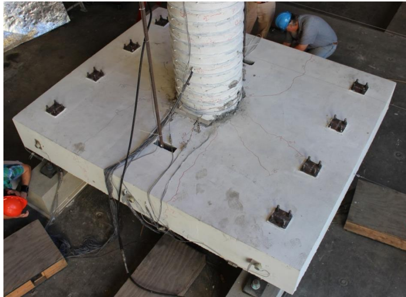
Figure 5.27 – Damage at the bottom face of the slab (top face in the specimen) of Specimen #1 at the end of testing
