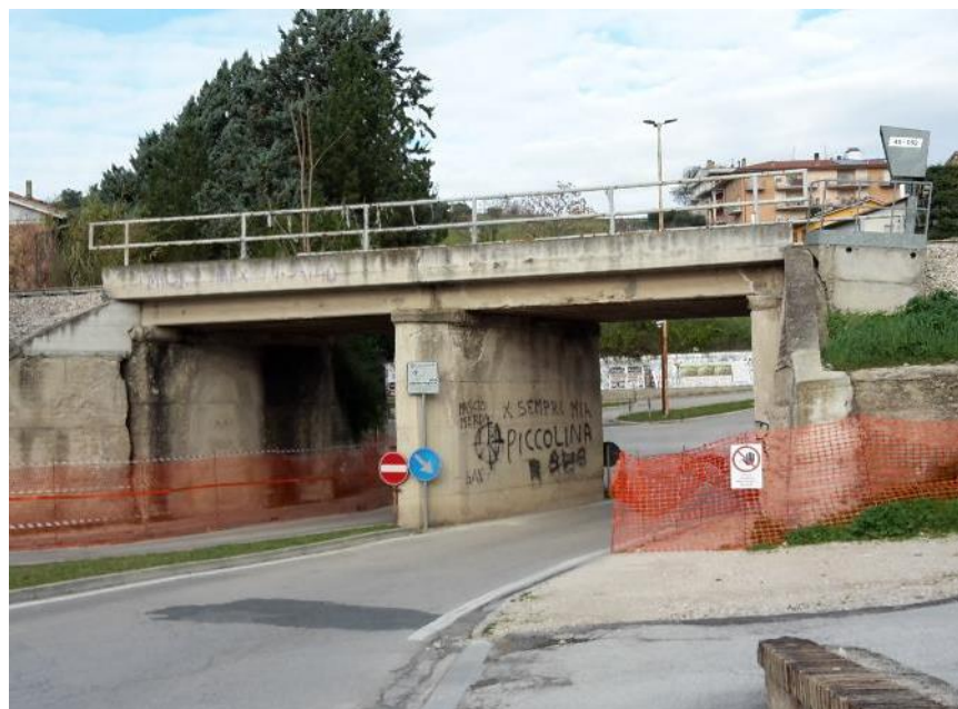
P12 (Damaged rail bridge)
