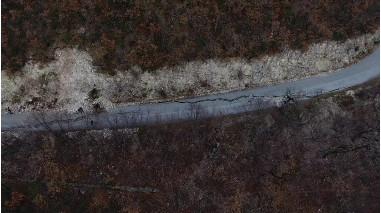
Figure 4.37. Landslide encountered along mountain road in the Valle di Panico (Point 5a).
