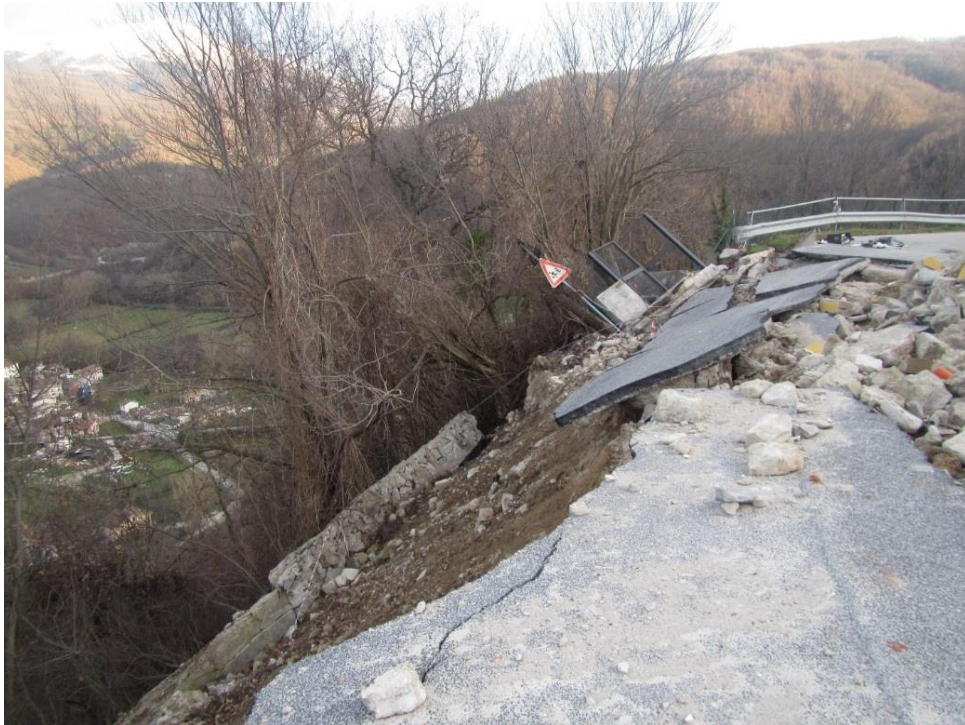
Figure 4.31. Failure of retaining wall due to shallow landslide (Point 4a, looking towards south).
