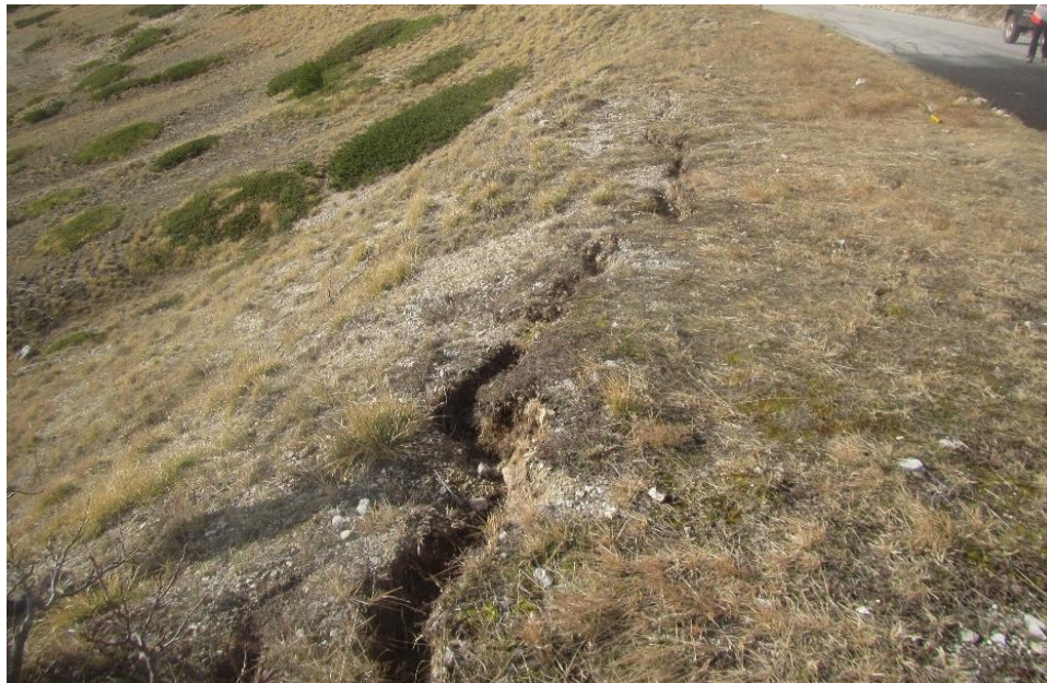
Figure 4.106. Road embankment damage along SP477 road, Mt Vettore (Location 19, viewing west).
