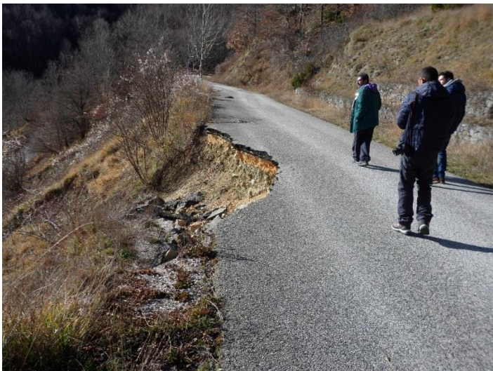
Figure 4.93. A slide observed on the fill slope.
