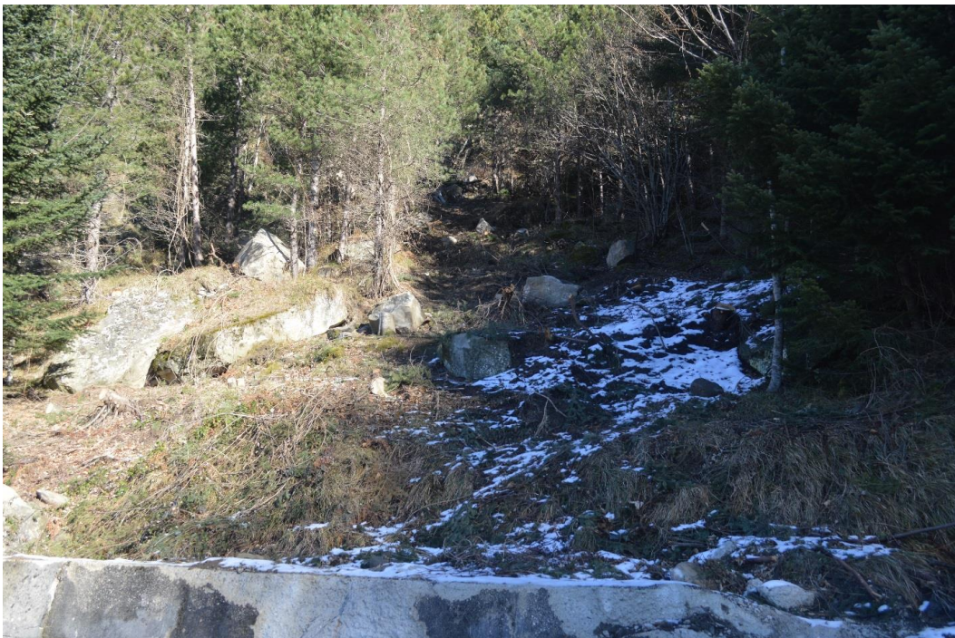
Figure 4.53. View upslope of damaged retaining wall, boulder fragments and runout chute from road at rockfall site near Crognaleto village.
