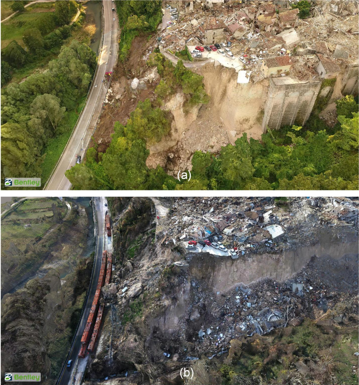
Figure 4.24. 3D model comparison of the failed retaining wall below Pescara del Tronto between September 2016 (a) and December 2016 (b).
