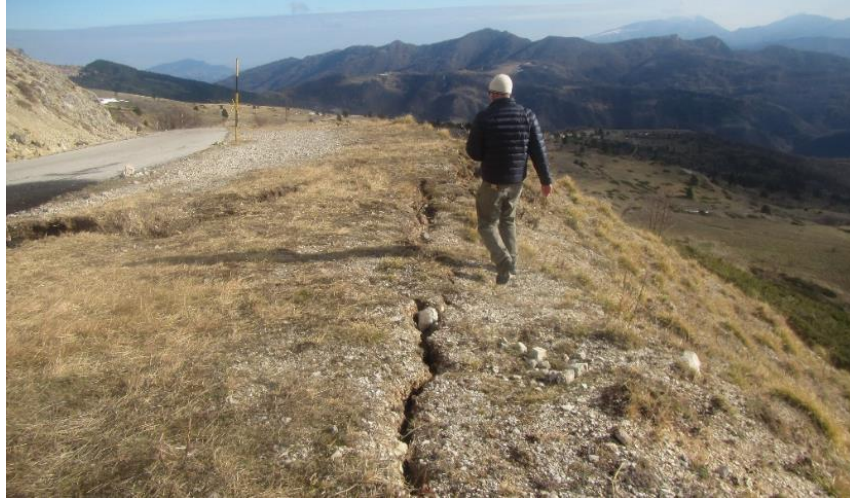
Figure 4.105. Road embankment damage along SP477 road, Mt Vettore (Location 19, viewing North). Note fault trace across road and black (new) bitumen repairs following previous (24 August 2016) earthquake.
