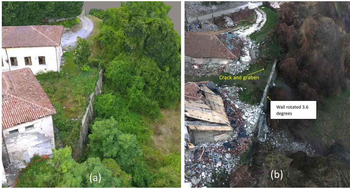
Figure 4.34. 3D model screenshots showing a retaining wall beneath the northeastern slope of Accumoli (a) undamaged in September 2016, and (b) damaged in December 2016.
