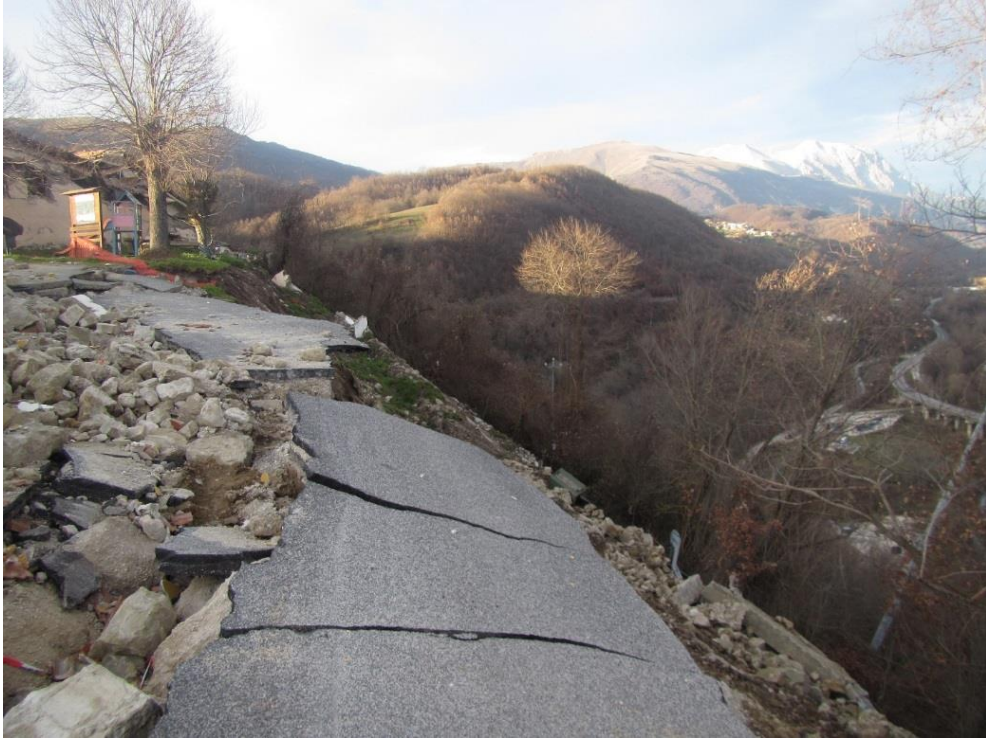
Figure 4.30. Failure of retaining wall due to shallow landslide (Point 4a, looking towards north).
