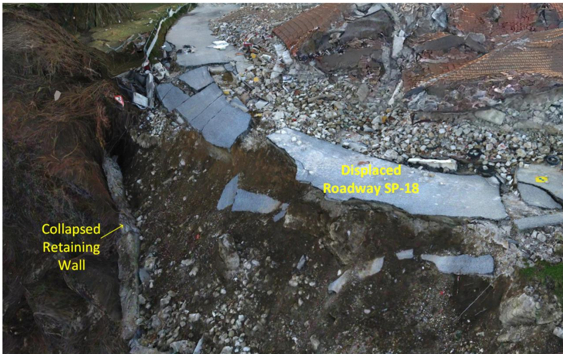
Figure 4.33. 3D model screenshot of the destroyed roadway Frazione Fonte del Campo (i.e., SP-18).
