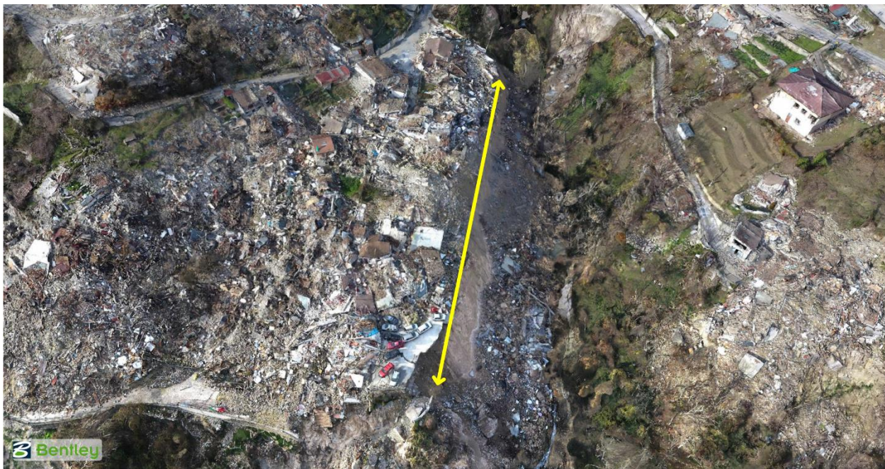
Figure 4.25. 3D SfM model view of scarp linearity behind failed lower retaining wall in Pescara del Tronto.
