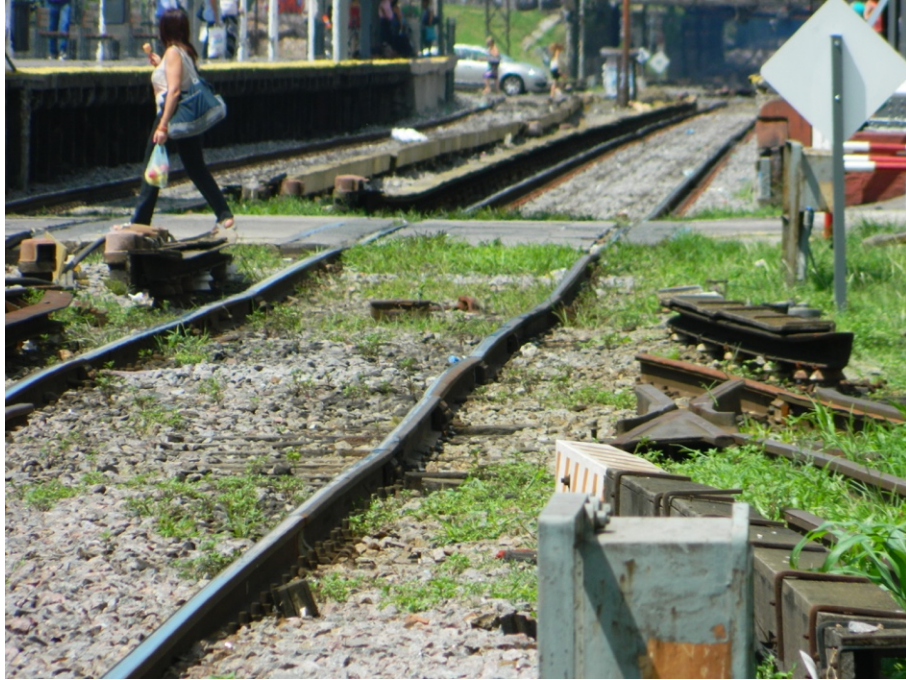
Figure 16: Deformed rails in Caballito station. Photo by author.
