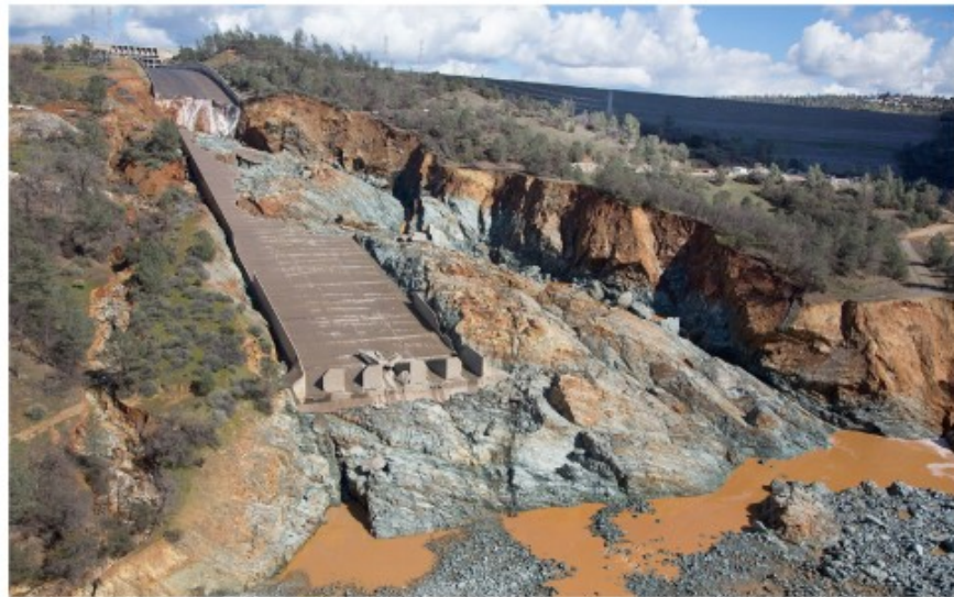
Fig. 1 Scour damage to service spillway at Oroville Dam in Northern California, 26 February 2017 (Kolke 2017)
