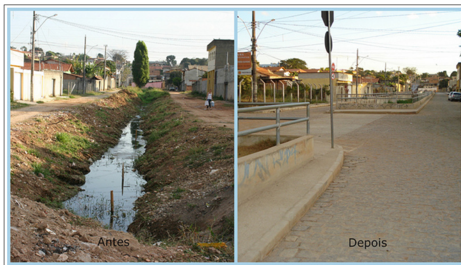
Figure 1.9: PB Sanitation Project - Before (Left) and After (Right): Pavement and sewer on Rua Gandhi, Belo Horizonte
