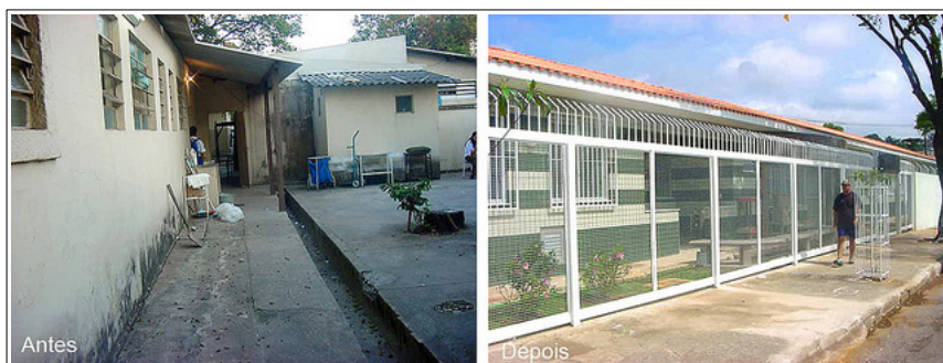
Figure 1.10: PB Health Project - Before (Left) and After (Right): Health center improvements (Centro de Saúde Tírol) in the region of Barreiro, Belo Horizonte
