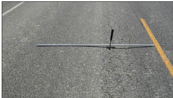
Figure 3.6: Rutting and fatigue cracking on a pavement with a cement-treated layer.
