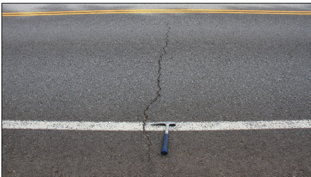
Figure 2.12: Early shrinkage crack in the vicinity of known cement accumulation.
