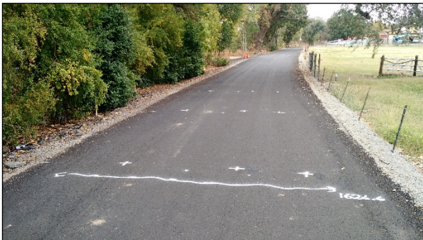
Figure 6.6: Marked crack with location.
