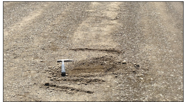
Figure 2.15: Sliver fill damaged by microcracking.
