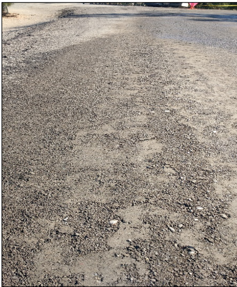
Figure 5.33: Surface damage after second microcracking effort at 72 hours.
