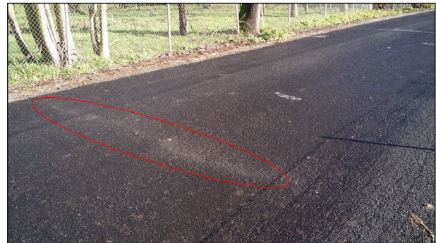
Figure 6.5: Crack identification by discoloration after water spraying.
