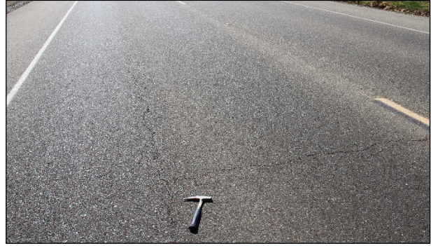
Figure 3.3: Longitudinal and transverse cracking on an FDR-C pavement.
