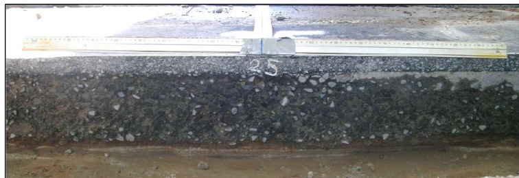
Figure 3.8: Disintegrated equivalent granular state of the cemented layer (17).
