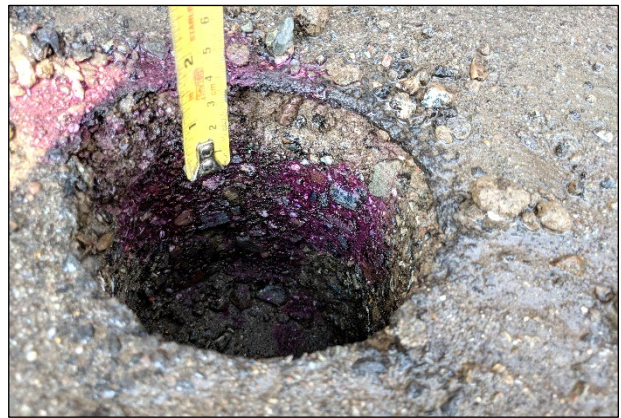
Figure 6.23: Carbonation with depth in core hole.
