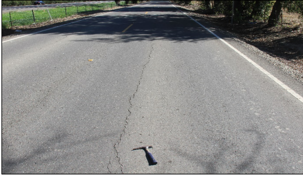
Figure 3.2: Longitudinal cracking on an FDR-C pavement.
