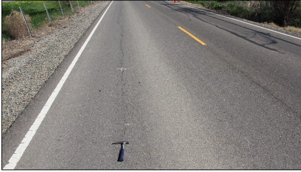
Figure 2.1: CR32B: Example longitudinal cracks.
