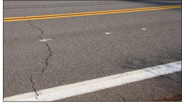
Figure 2.5: PLU-147: Example transverse crack.
