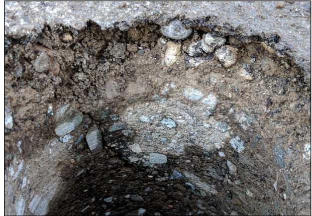
Figure 6.26: Disintegration of FDR-layer surface attributed to carbonation (side view).
