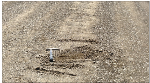
Figure 2.15: Sliver fill damaged by microcracking.
