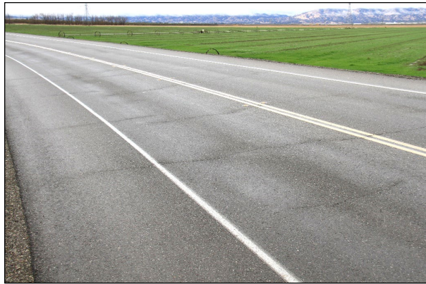
Figure 3.1: Reflected shrinkage cracks on a pavement with an FDR-C base.
