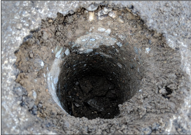
Figure 6.25: Disintegration of FDR-layer surface attributed to carbonation (vertical view).
