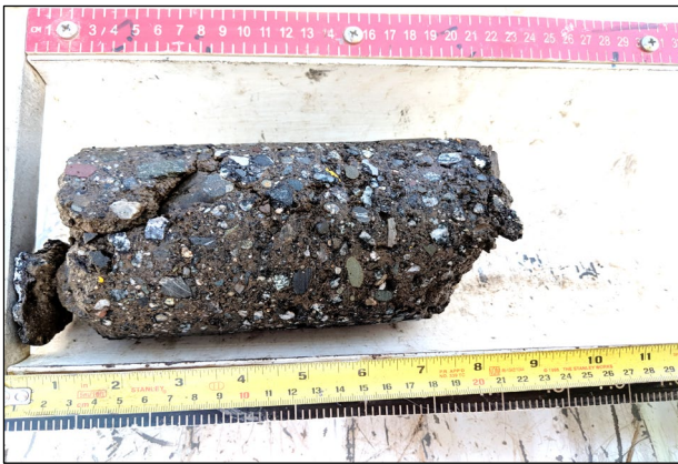
Figure 6.22: Core taken across shrinkage crack.
