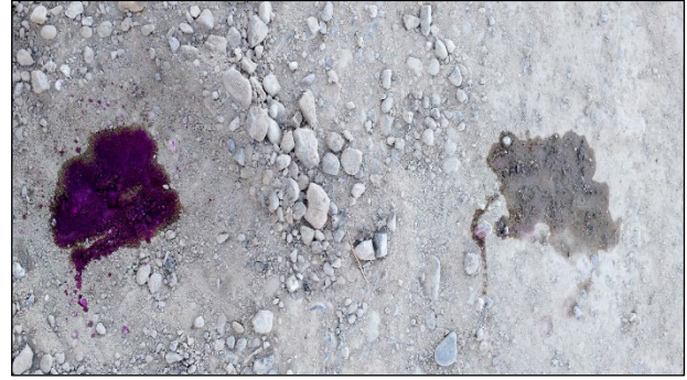
Figure 2.17: Carbonated area (no color in sprayed area) attributed to inappropriate curing.
