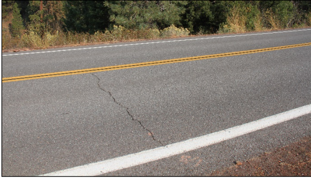
Figure 2.4: PLU-147: Example transverse crack.
