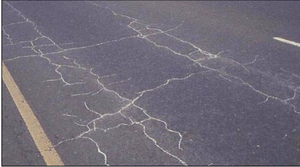
Figure 3.4: Block cracking on an FDR-C pavement (note pumping of fines through cracks).
