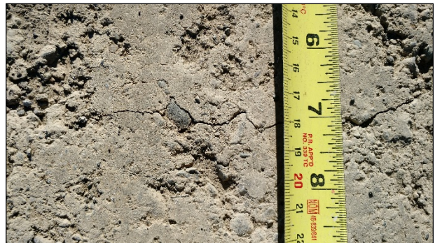
Figure 6.9: 4% Cement: Shrinkage crack width on Cell S9 after 48 hours.
