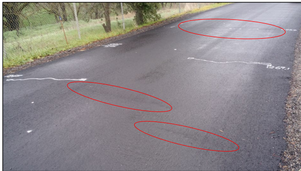
Figure 6.4: Crack identification by differential drying after water spraying.
