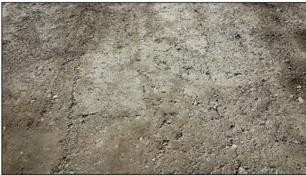
Figure 2.14: Block cracking after microcracking in known area of cement accumulation.
