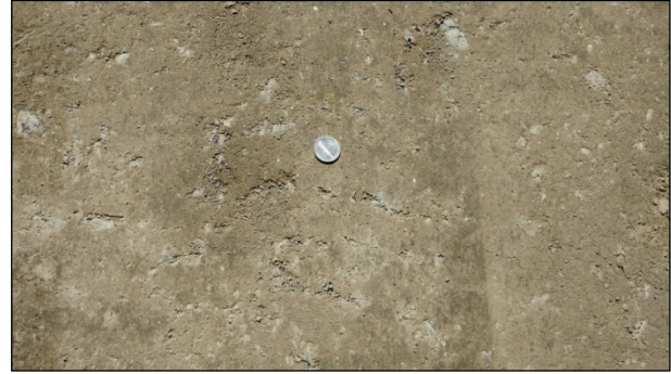
Figure 5.32: Close-up of microcracked surface.
