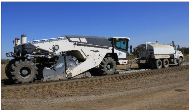
Figure 5.6: Water tanker and reclaimer.
