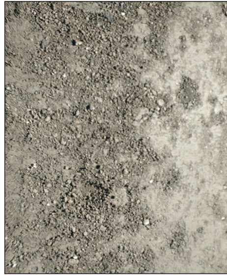
Figure 5.34: Close-up of surface damage after second microcracking effort at 72 hours.
