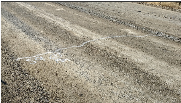
Figure 6.8: 4% Cement: Shrinkage crack on Cell S9 after 48 hours.
