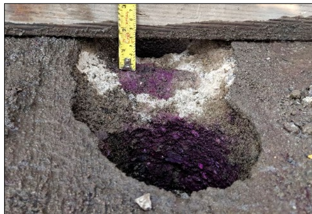
Figure 6.24: Carbonation extent beneath microsurfacing.
