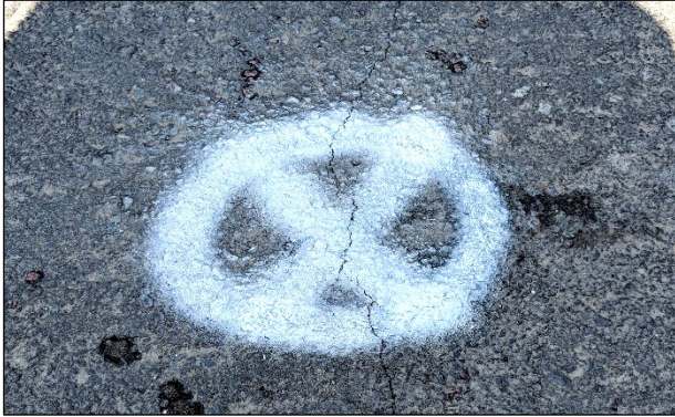
Figure 6.20: Core location through shrinkage crack.
