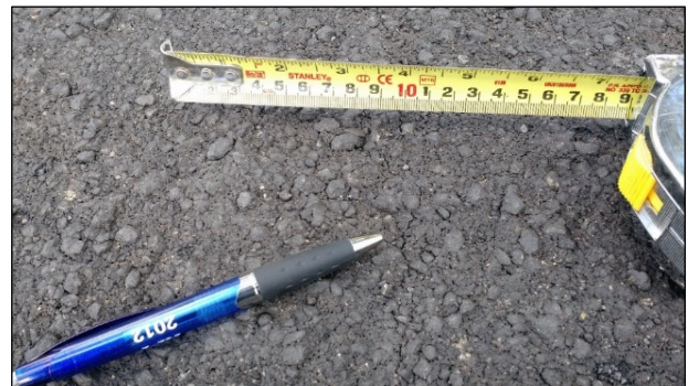
Figure 6.2: Narrow crack width of drying shrinkage crack at first appearance.
