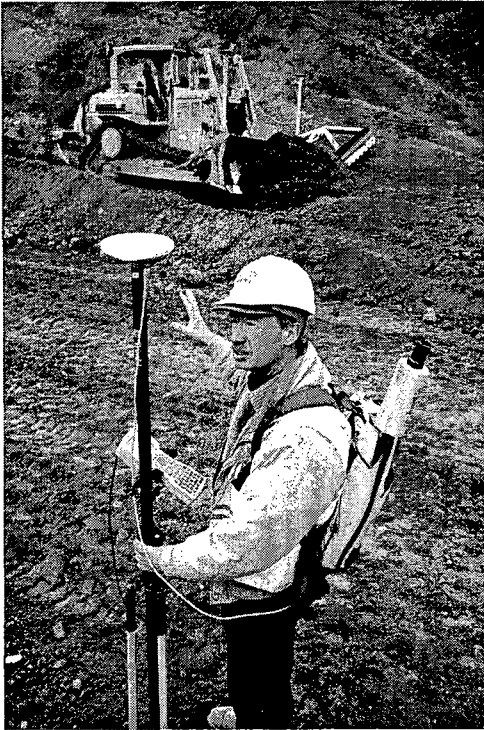
Ghilotti engineer Rich Faria carries GPS surveying gear. Vertical poles on the bulldozer blade are GPS antennas. (Photo by Robert Couto)
