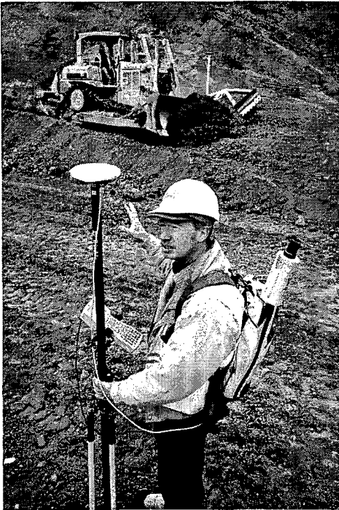
Ghilotti engineer Rich Faria carries GPS surveying gear. Vertical poles on the bulldozer blade are GPS antennas. (Photo by Robert Couto)
