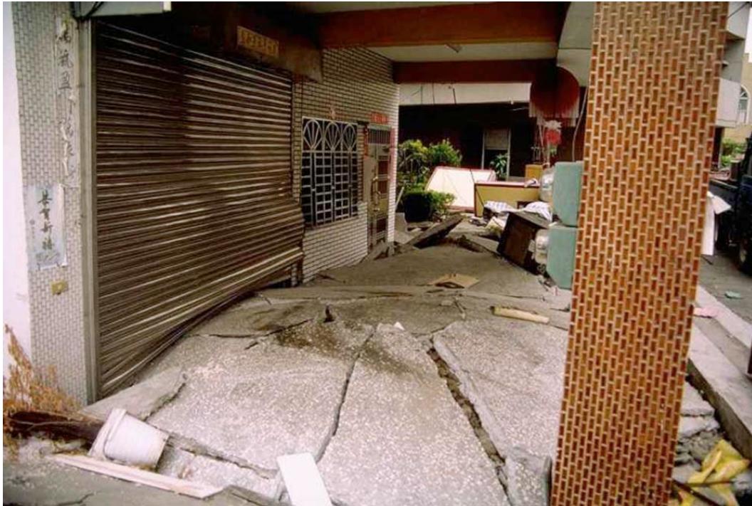
Fig. 1 – Punched footings and intermediate slab heaving due to cyclic softening of high-plasticity clay in Wufang, Taiwan. Photo by R. Seed (1999).
