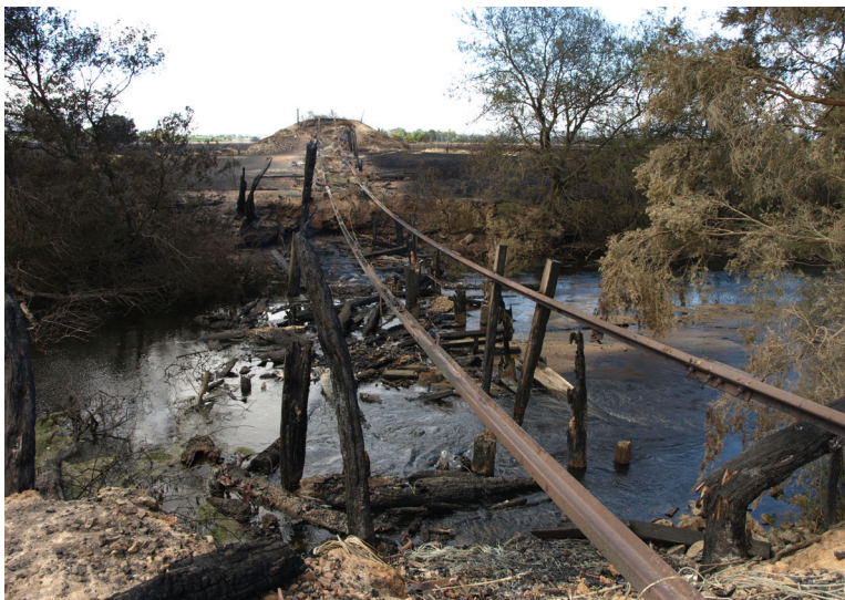
Figure 1: Railway track and bridge destroyed by the Black Saturday firestorm outside Melbourne, Australia, February 2009. Source: Adam Taylor
