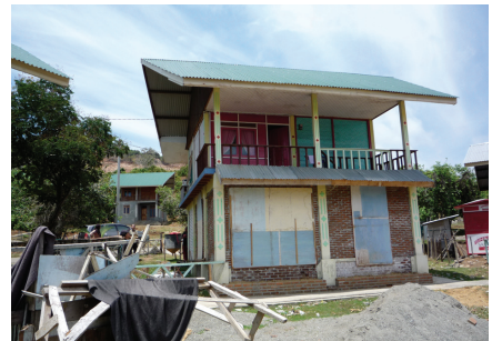
Figure 3: The residents of this Bank Mandiri house are in the process of enclosing the undercroft space to provide a new kitchen and living area. Progress is slow and until further finances can be generated the proposed windows have been blocked with sheets of plywood
