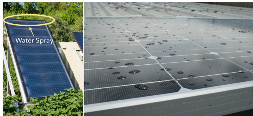
Figure 5. PV cells shown in use, with water cooling system attached on the top end of the set-up. Spraying of water on the surface of the cells helps cool them. (image courtesy: Dominic Alves)
