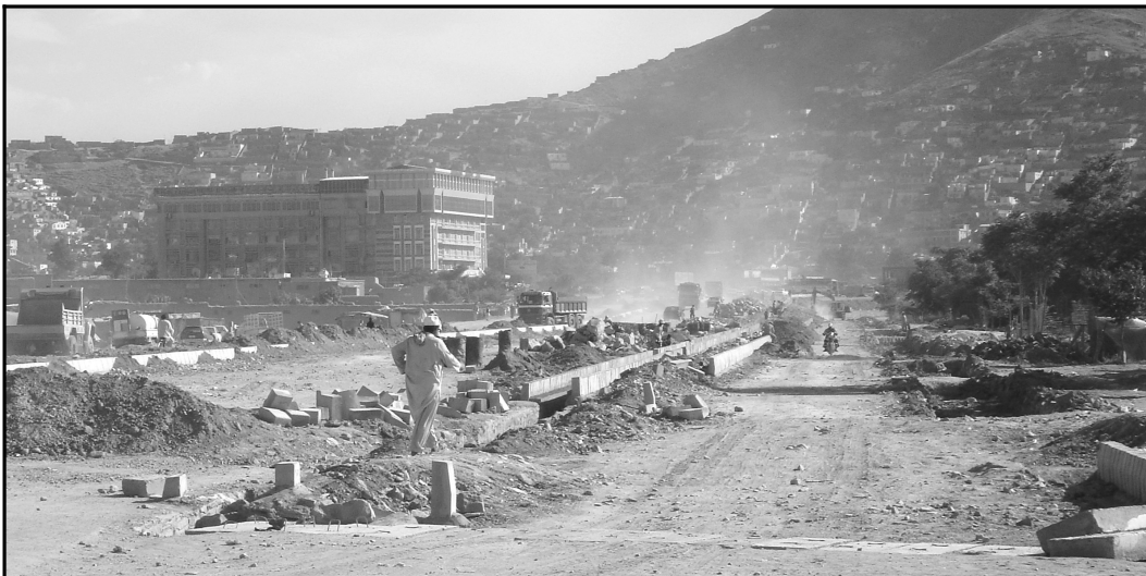
Figure 4.32. Sixty-meter roadway under construction near Kart-e Parwan (author, 2007). Note both the new office building and the informal housing in the background.
