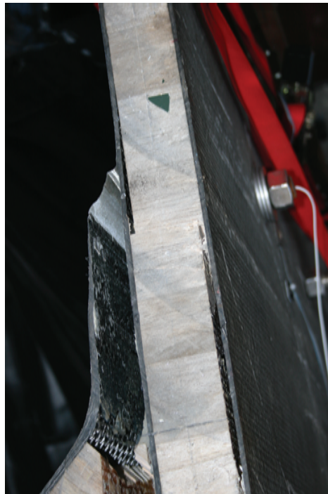
Figure 3.105: Photo of post damage in Composite Joint Test 5.
