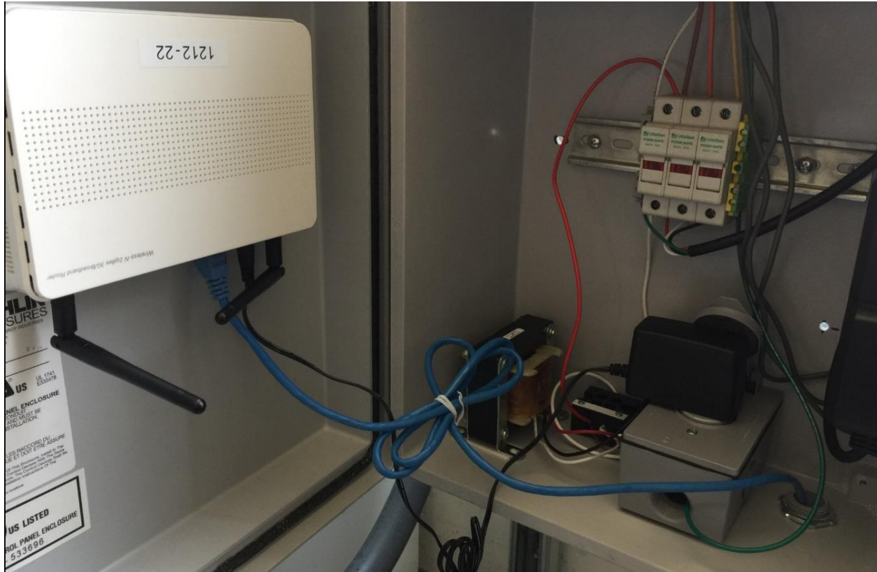
Figure 44. Inside view of the network equipment box
