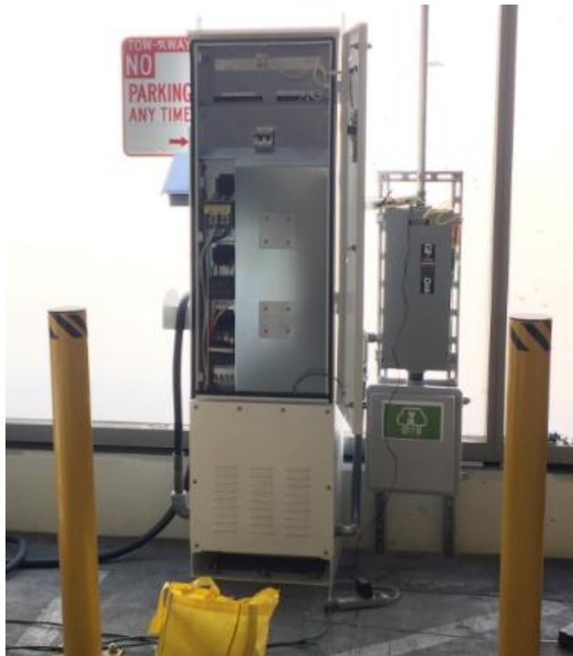
Figure 43. Network Communication equipment box
