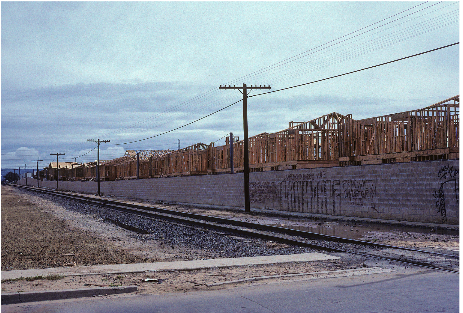
New homes under construction alongside the Santa Fe Harbor District in Lawndale, April 1983. A sound wall constructed by the developer shields only the bottom floor. The author visited a display home and asked the real estate agent about train traffic behind the homes. She replied, "Oh, they don't run on that line much anymore." (Yeah, right.)
