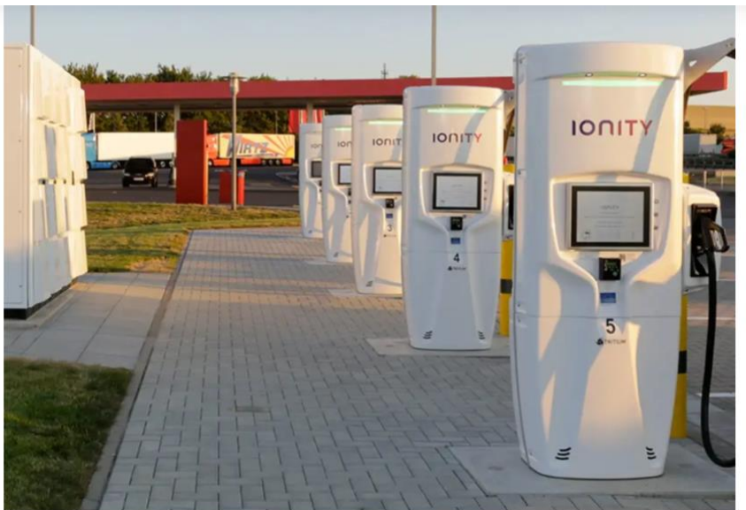
Figure 14. A rectifier with multiple chargers
