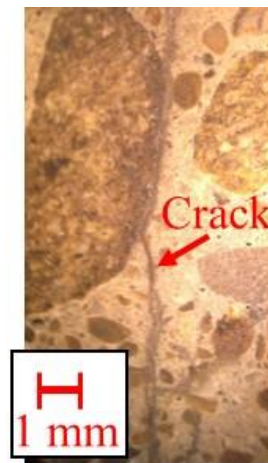
Figure 31: A isolated splitting crack for OC-C(0.75)
