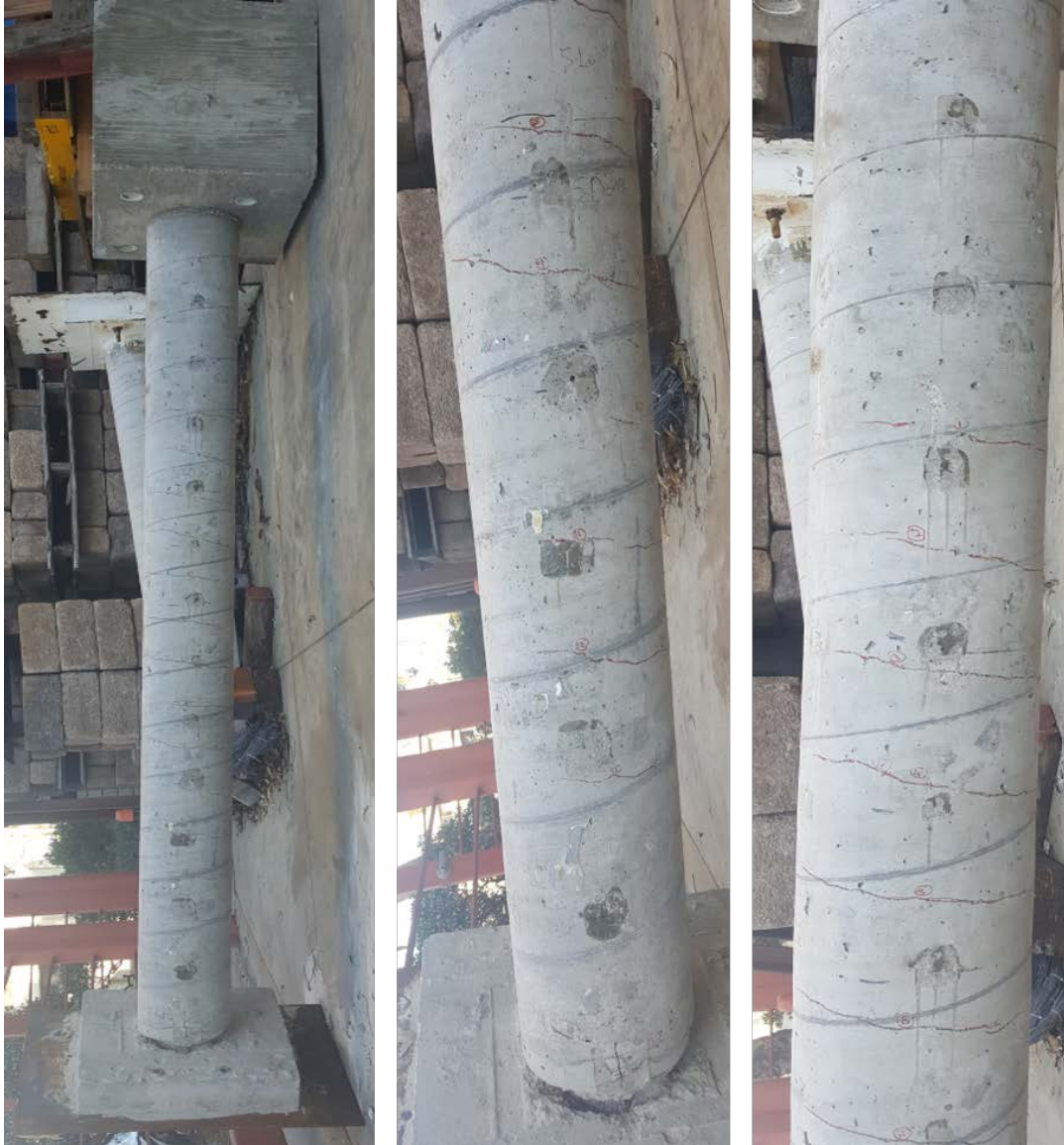
Figure 9-25. Observed breakage of the concrete pile at the base and cracking along the height
