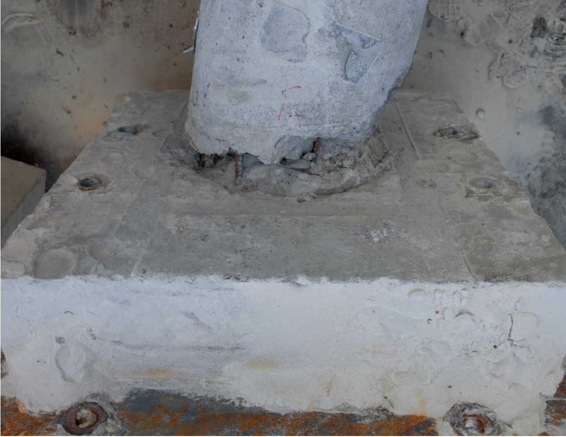
Figure 9-26. Pile breakage at the base
