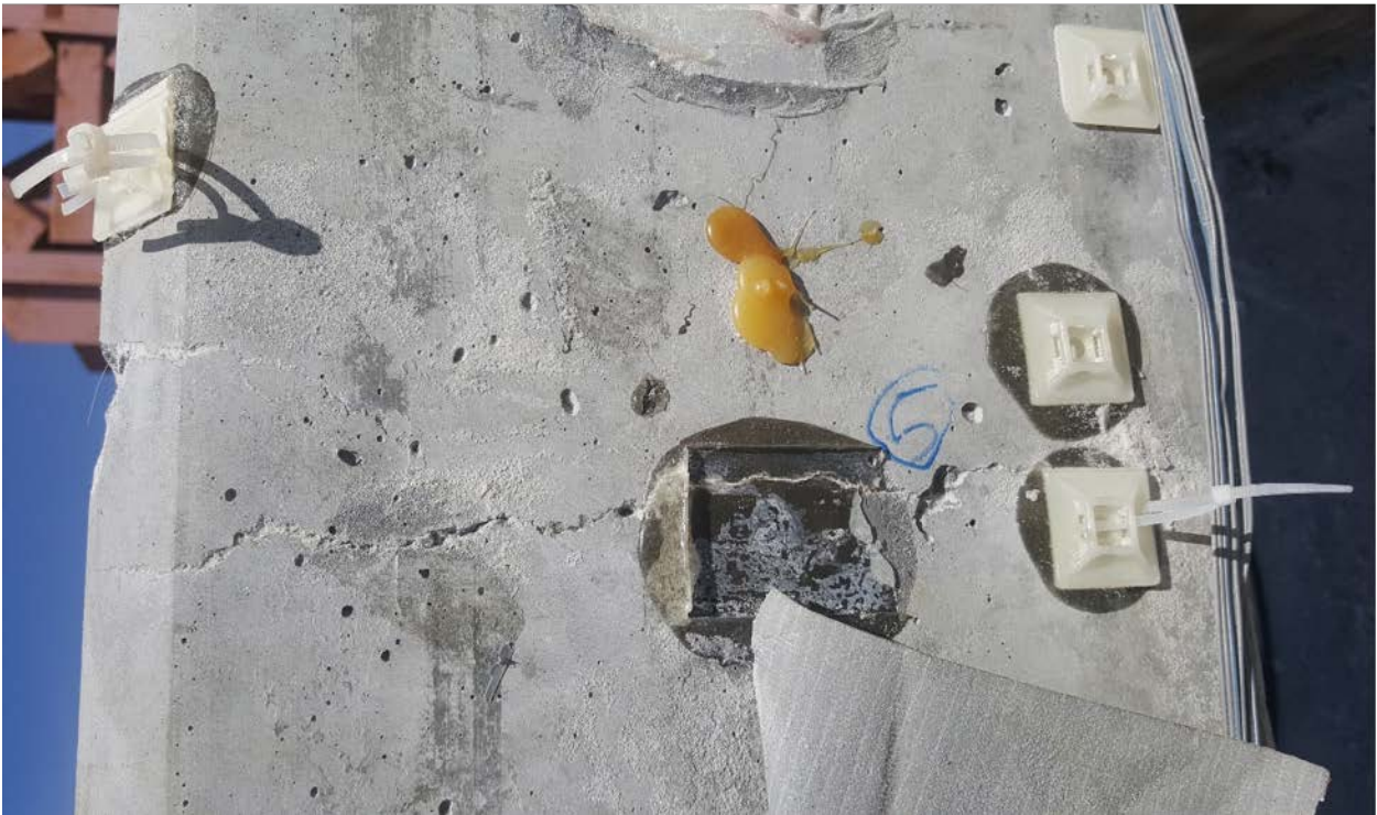
Figure 11-33. Picture of pile cracking
