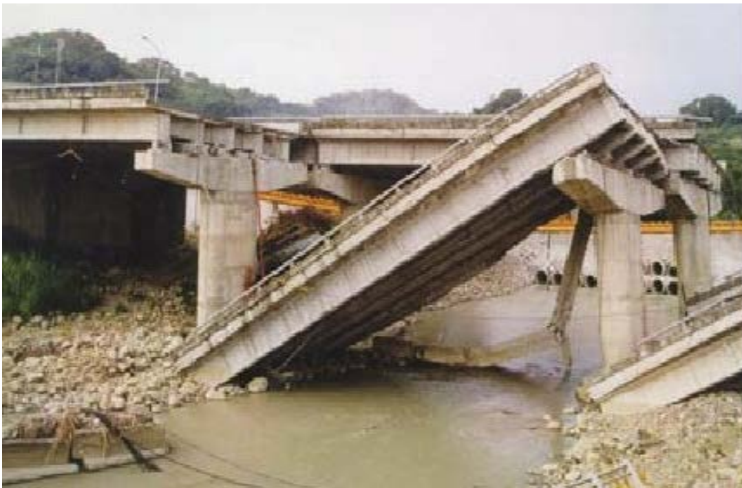
Figure 1-12. Collapse of a bridge by excessive lateral movement during the 1999 Chi-Chi Taiwan earthquake (after Moehle and Eberhard 2000)
