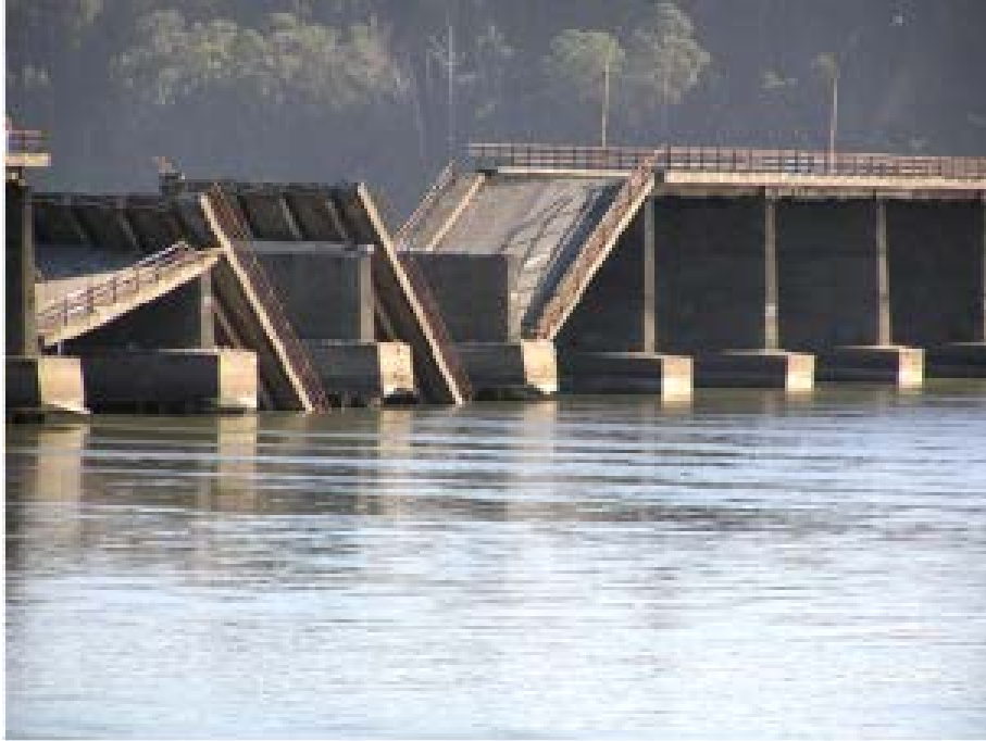
Figure 1-15. Collapsed decks caused by lateral spreading, Photo by Scott Brandenburg (GEER Association Maule Chile 2010a)
