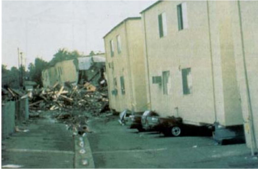
Fig 1.4: Total collapse of soft storeyed open garage at the ground floor of the apartment building in Northridge earthquake
