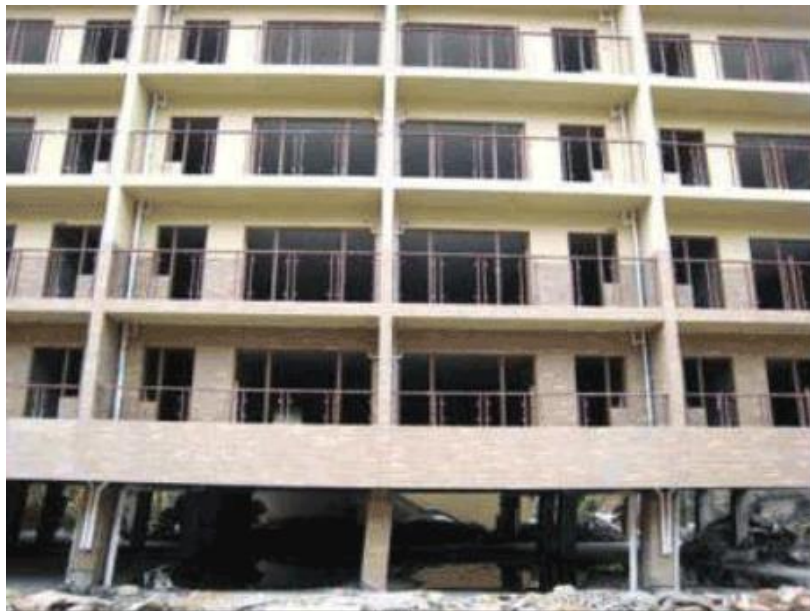
Fig 1.3: A six storeyed building with soft-storeyed ground floor at Dujiangyan in 2008 China earthquake
