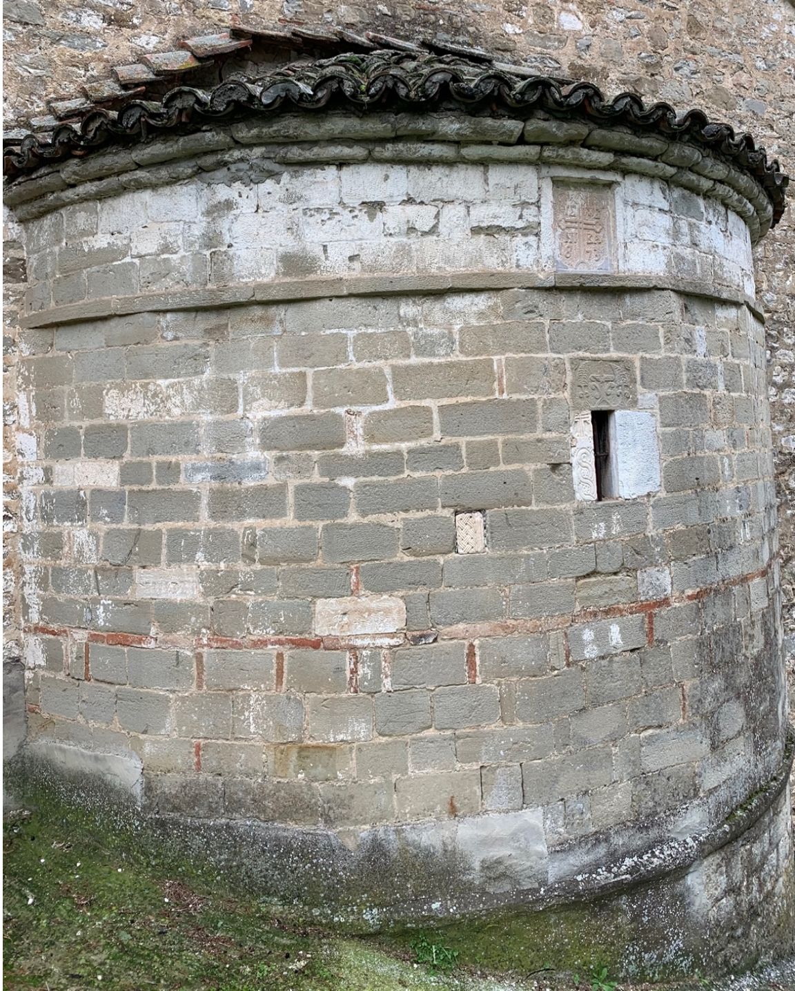
Figure 18. Church of Agios Ioannis Prodromos, at Fanari, 1873. East façade. Photograph courtesy of the author.
