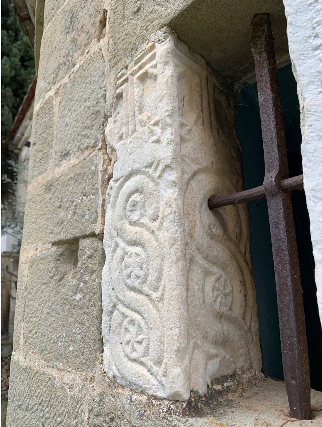
Figure 20. Church of Agios Ioannis Prodromos, at Fanari, 1873. Marble fragment from east façade. Photograph courtesy of the author.
