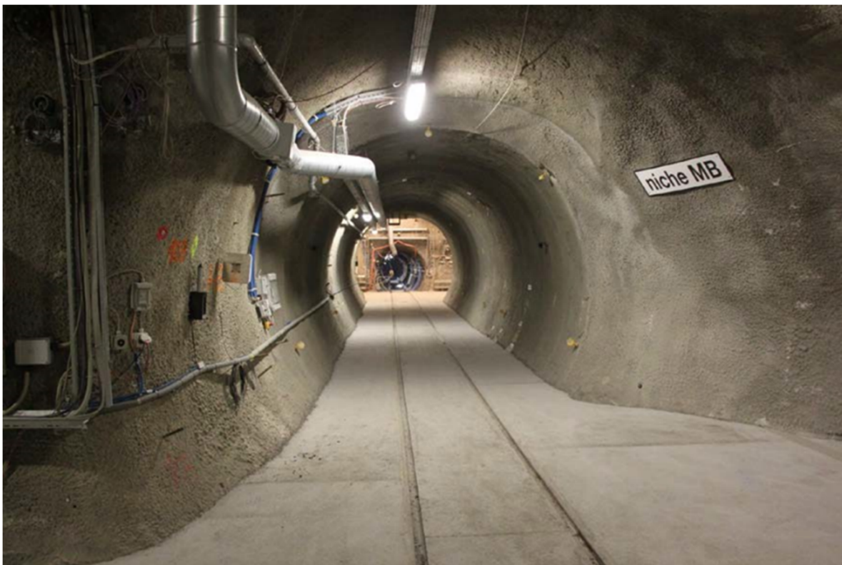
Figure 3.1-7. View from the FE gallery into the heater tunnel during final installation (Bossart, 2014).
