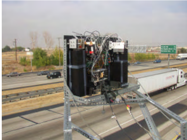
Figure 5-3. Detection system mounted above the highway
