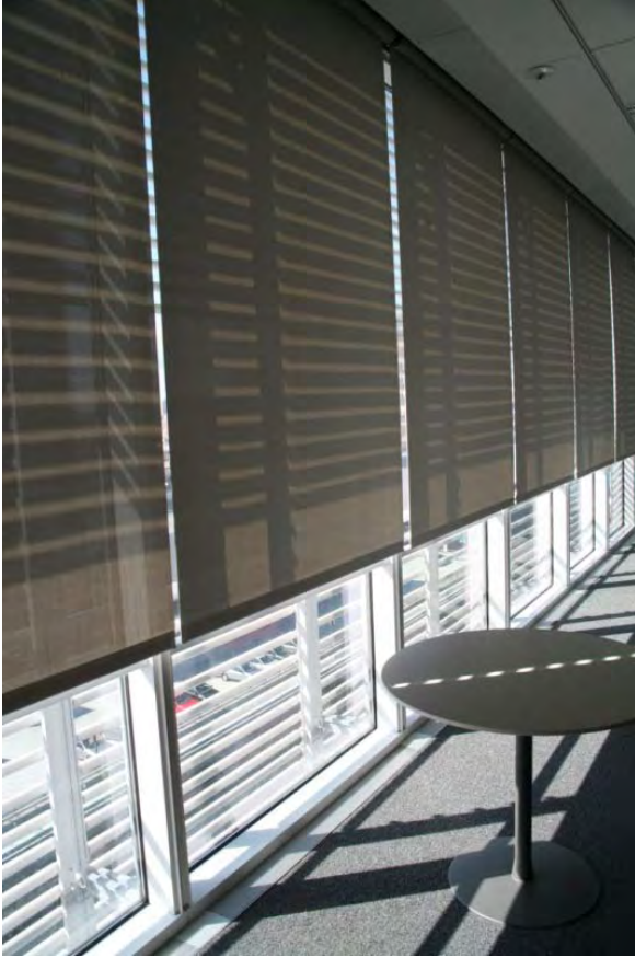
Figure 13. The automated shades controlled direct sun to within 3 ft from the window wall at floor level in most open plan work areas. Copyright: LBNL.
