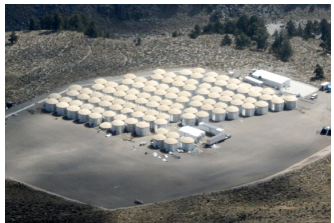
Figure 1: May 16, 2013 picture from the HAWC site. Steel from approximately 30% of the final WCDs are visible. The cleared area indicates the size of the completed instrument, \sim 20000\text{ m}^2 .
