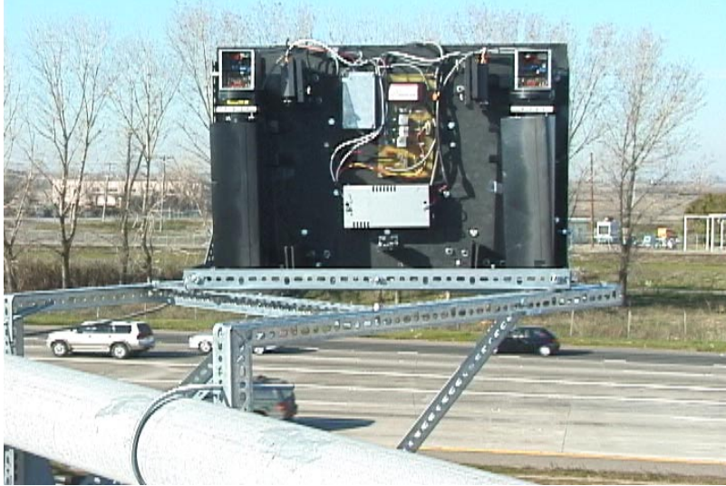
Figure 8-4: Detection System Mounted Above the Highway.
