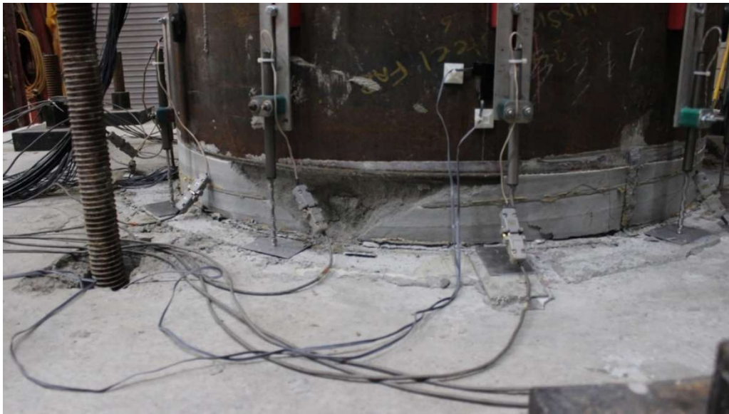
Figure 9.41: Picture of spalling on south side of Specimen 2 after first cycle at 0.83% drift ratio
