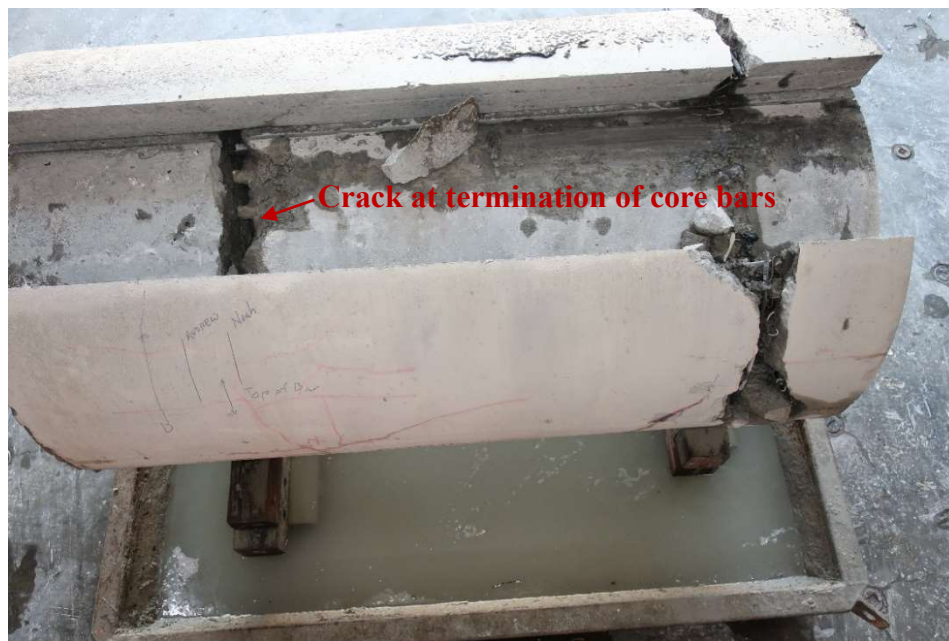
Figure 4.25: Exposed core after the shell was partially removed from Specimen 2 showing a through crack in the core near the termination point of the core bars
