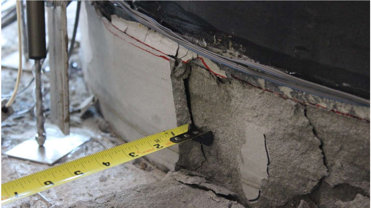
Figure 9.8: Picture of south side of Specimen 1 at peak drift of 5.01%
