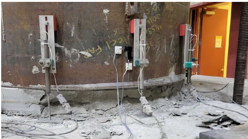
Figure 9.42: Picture of spalling on south side of Specimen 2 after first cycle at 2.51% drift ratio
