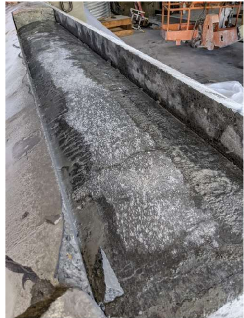
Figure 4.43: Pictures of exposed concrete core of Specimen 3 showing a crack at 13 inches from the soffit of the pile cap (shell removed during demolition)
