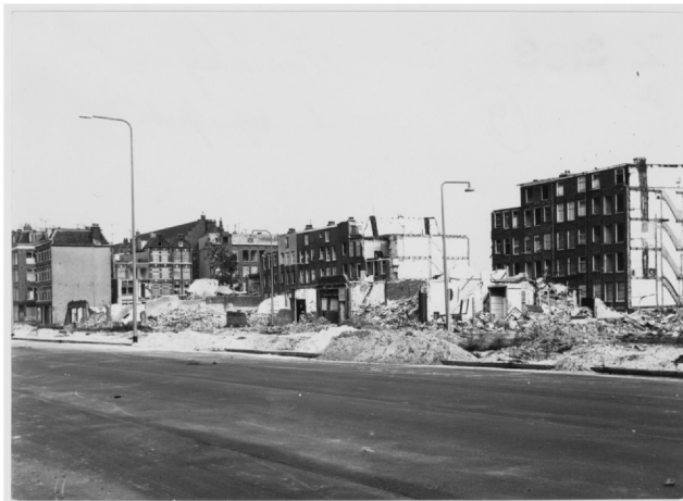
Fig. 7 Photo of the beginning of the demolition and construction of Grote Kattenburgerstraat. Stadsarchief Amsterdam (1967 ca.) Kattenburg, links begin Grote Kattenburgerstraat. Sloop, Gemeente Amsterdam Stadsarchief. [Photo]. https://archief.amsterdam/beeldbank/detail/c85ff8e5-5ddf-68c4-45f0-dae550c548aa .
