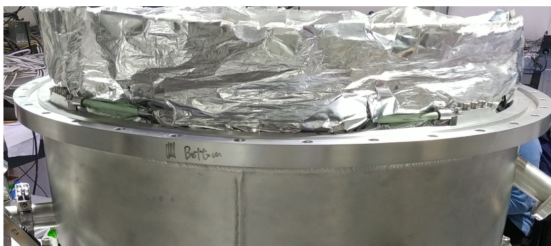
Figure 2.22: This photo shows the new OT struts installed between the 4 K and 50 K shells at the aperture lens.
