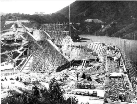
Figure 3.1. Two reservoirs under construction in Hong Kong, early 1900s. (Source: The National Archives of the U.K.: Public Records of Office, London).
