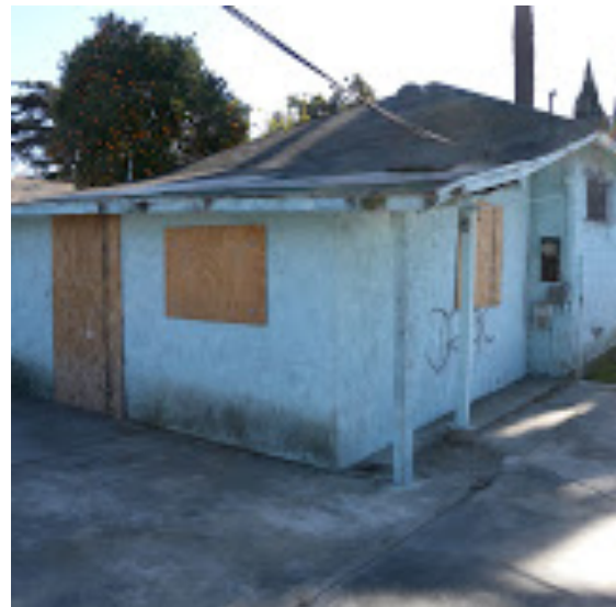
City of Los Angeles, 113 th Ave, 90059 – Before Construction. Courtesy of the Los Angeles Housing & Community Investment Department (HCIDLA).
