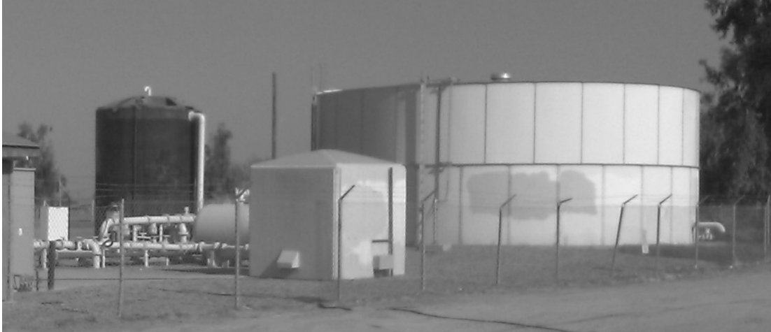
Figure 75: Water treatment plant in Lanare, California (contemporary photo by author).
